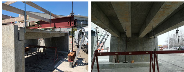
Fig. 5 Static load test setup: on the left is shown the static loading system
