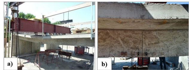
Fig. 17 Residual deformation experienced at the end of the load test (a) and the observed crack pattern (b)
