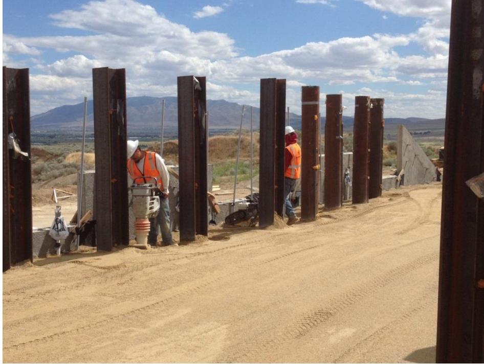
Figure 3.10: Jumping jacks for compaction around test piles and vibratory plate for compaction within 3 ft. of wall.
