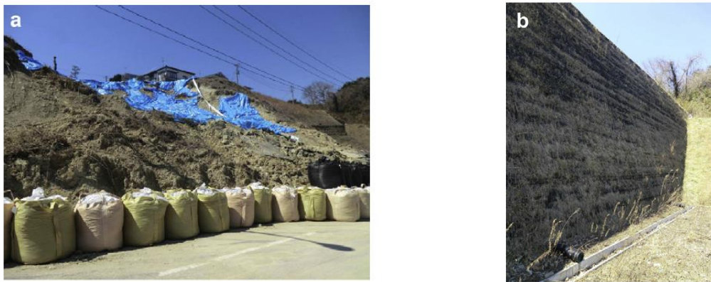
Figure 2.5: (a) Collapse of unreinforced embankment and (b) undamaged GRS RW at Yamamoto town, Miyagi (Koseki 2012).
