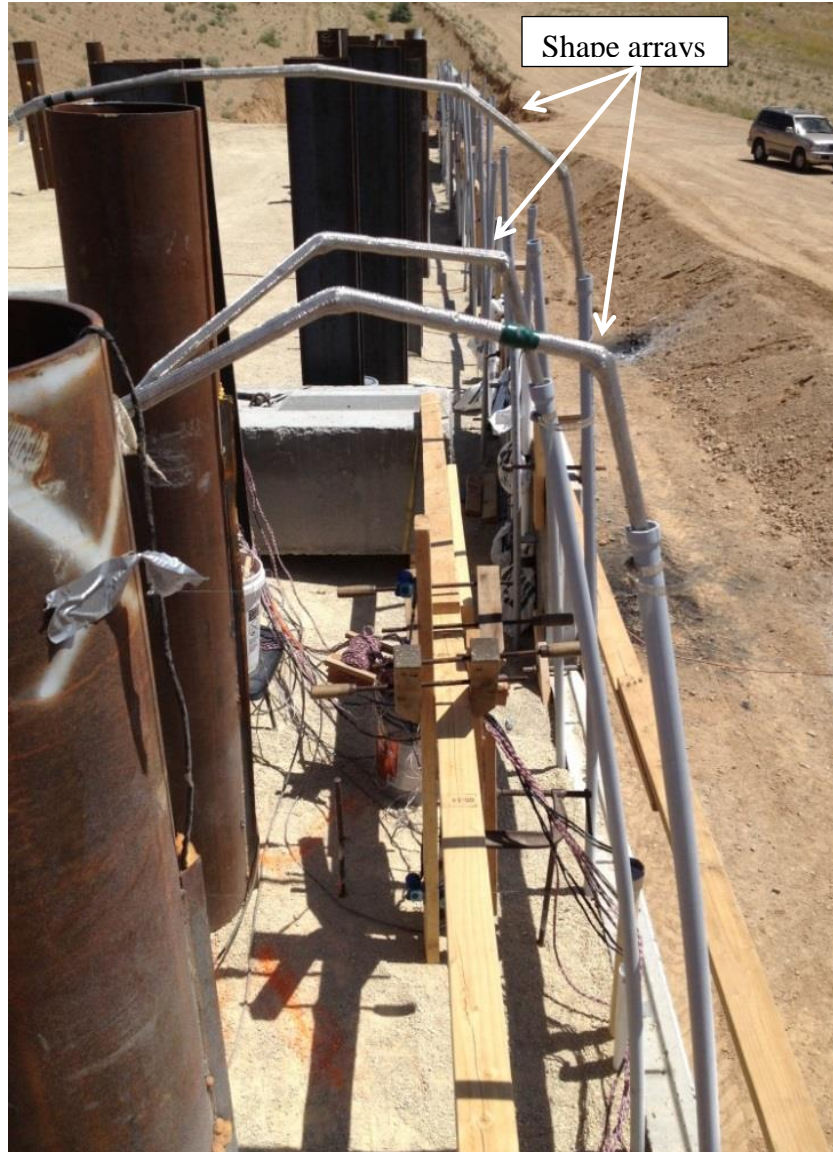
Figure 4.12: Photograph of shape arrays in place behind the face of the wall.
