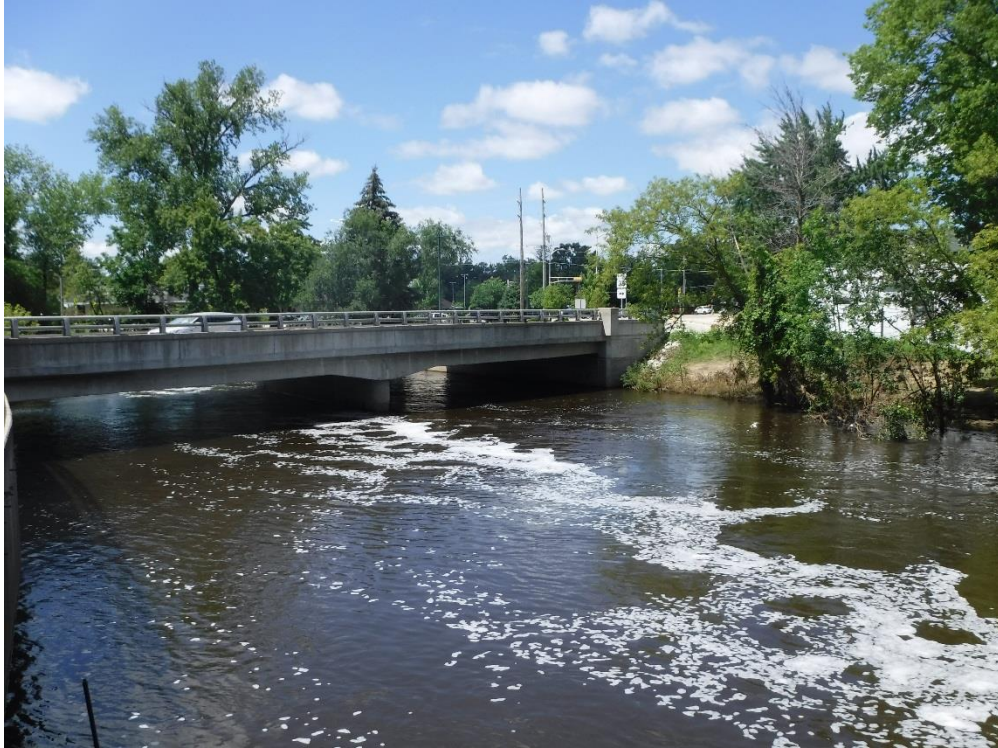
Figure 10: Minimal clearance between highwater surface and superstructure low chord
