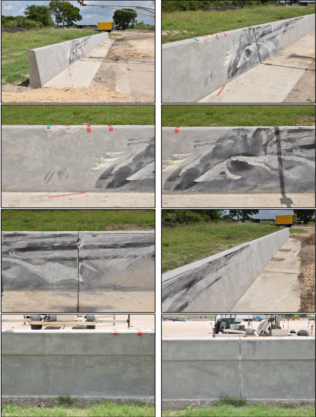
Figure 6.3. Barrier after Test No. 469689-3-3.
