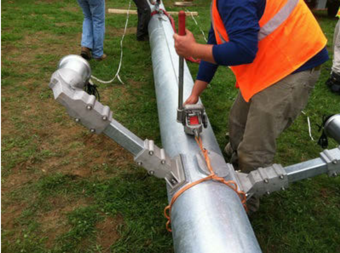
Figure 7. Multiple CLDs Attached to a Single Pole (Image courtesy of MG 2 )
