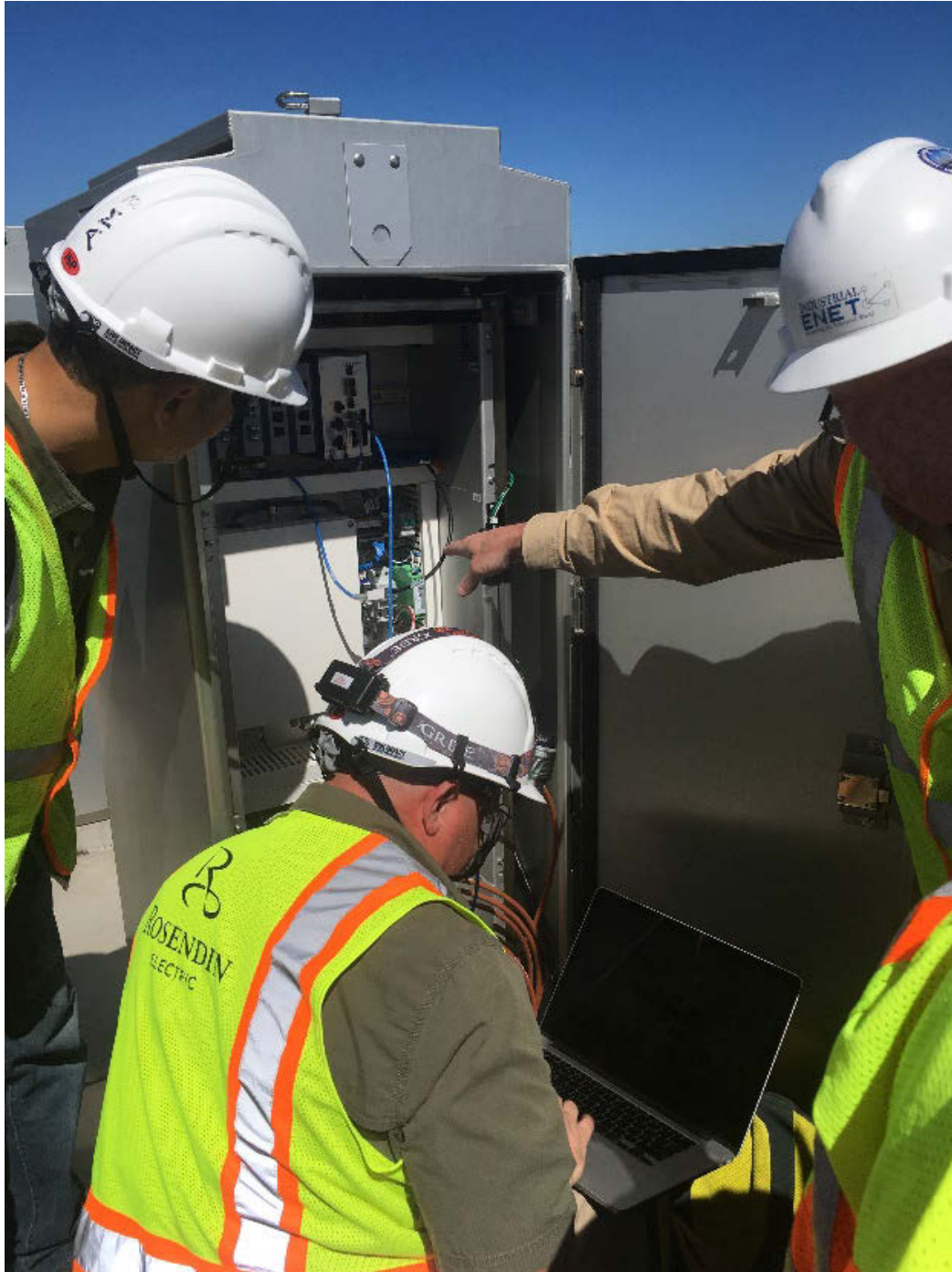
Figure 60. Bay Bridge MG2 CLD Remote Eletronics Cabinet
