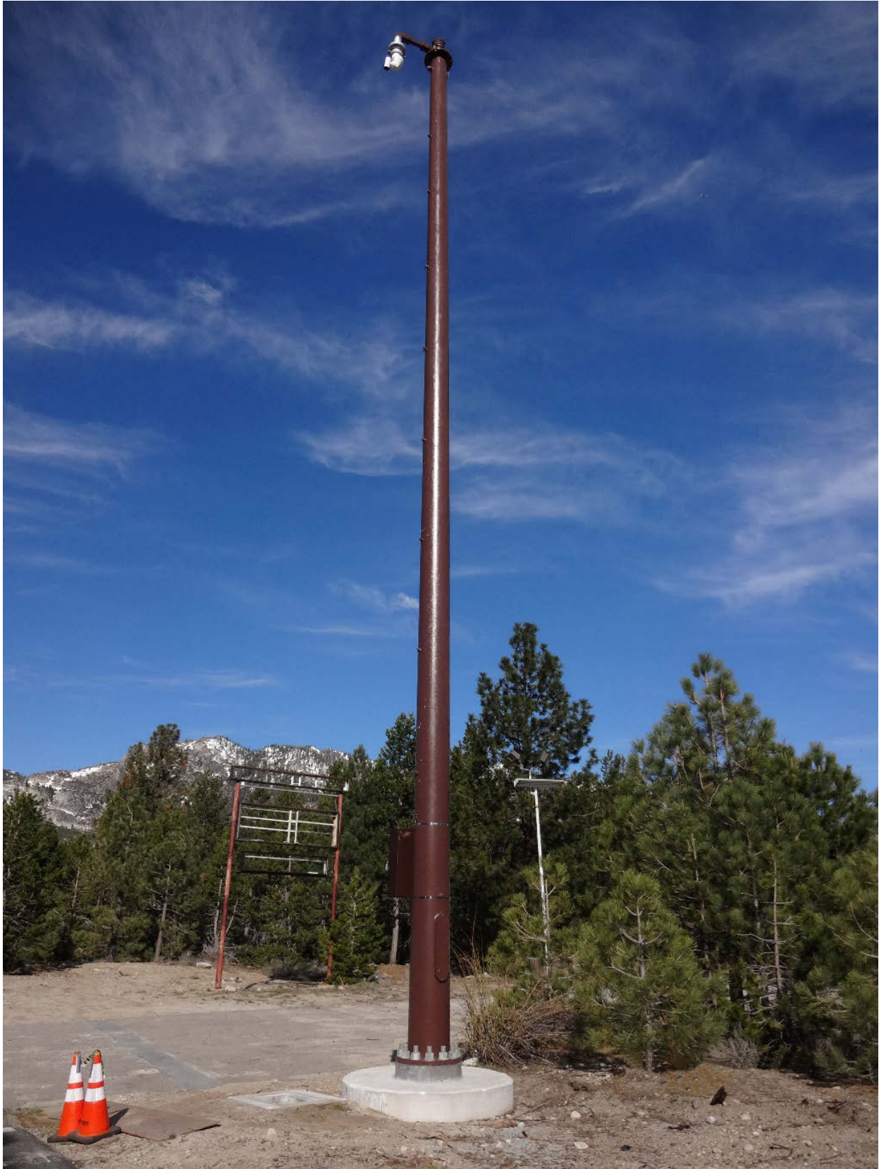
Figure 48. As-Built Meyers MG 2 Internal-type CLD Site
