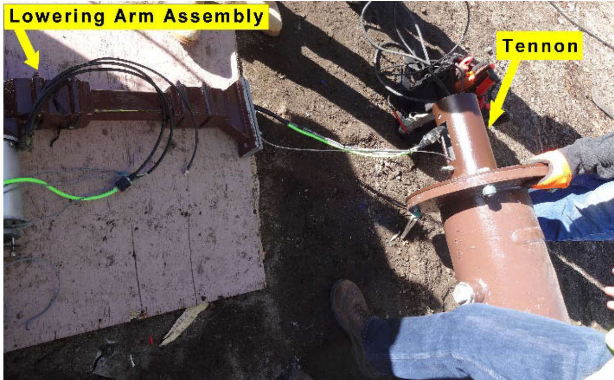
Figure 31. Pole Tenon Electrical Connections
