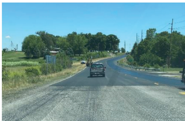
Figure 2.2 U.S. 421 project west of Delphi, IN—typical milled surface used for driving surface.
