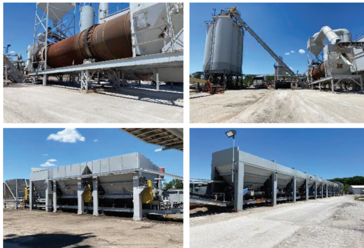
Figure 2.5 Hot mix plant used for asphalt mixture on U.S. 421. Clockwise from top left, embedded burner drum mixer, silos with drum mixer and drag slat, aggregate cold feed bins, and RAP cold feed bins.
