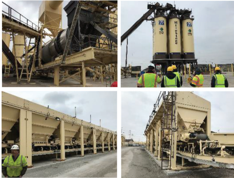
Figure 2.28 Hot mix plant used for asphalt mixture on SR 135. Clockwise from top left, embedded burner drum mixer, silos with drum mixer and drag slat, aggregate cold feed bins, and RAP cold feed bins.
