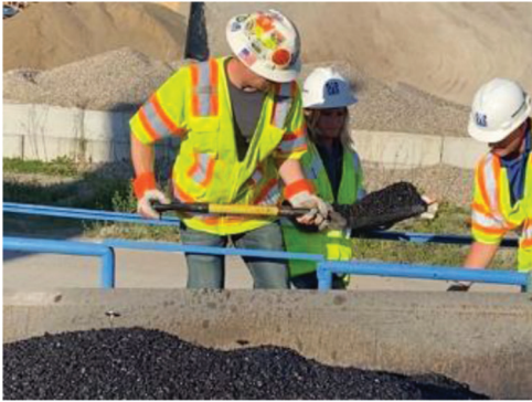
Figure 2.7 Plant-mix sample for the 12.5-mm intermediate mixture that was taken from a truck box at the sampling stand of the hot mix plant.
