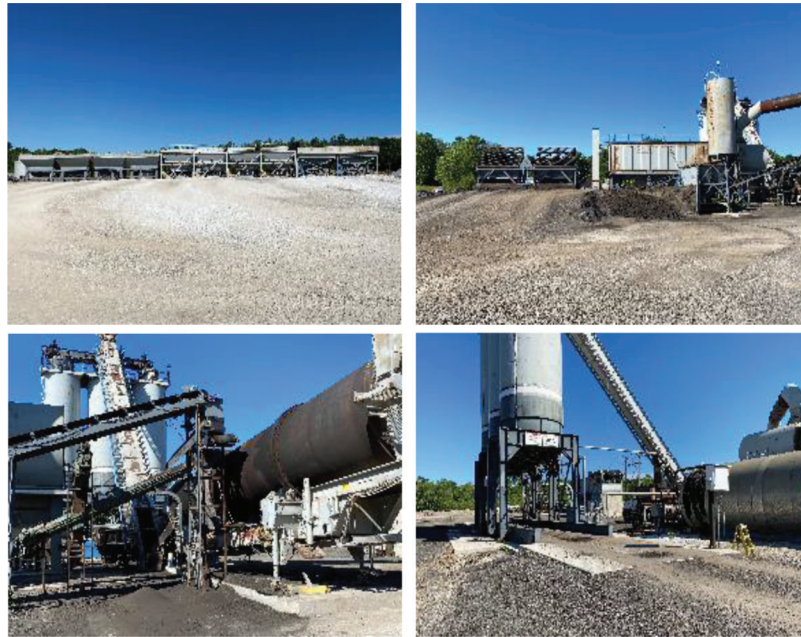
Figure 2.19 Hot mix plant used for asphalt mixture on U.S. 231. Clockwise from top left, embedded burner drum mixer, silos with drum mixer and drag slat, aggregate cold feed bins, and RAP cold feed bins.
