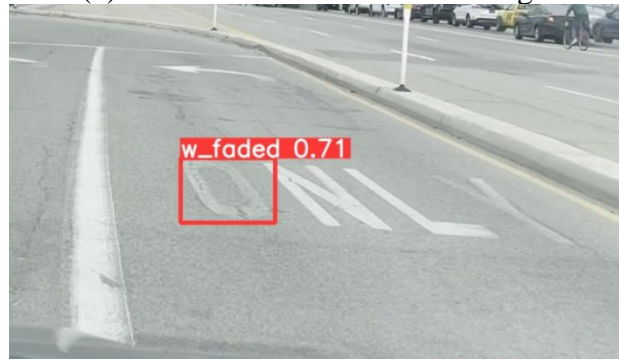
(f) Faded white delineator markings
