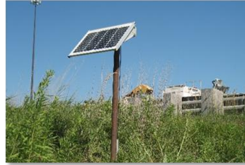
(b) Solar panel
