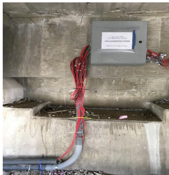
Figure 5.13. Wires to DAS
