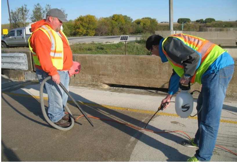
Figure 5.3. Crack survey using wet test method (water used to wet concrete surface)
