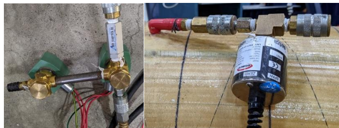
Figure 22. Air pressure regulator and transducer
