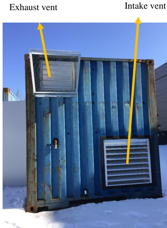
Figure 2.5: Intake and exhaust vents of duct system on the exterior of container.
