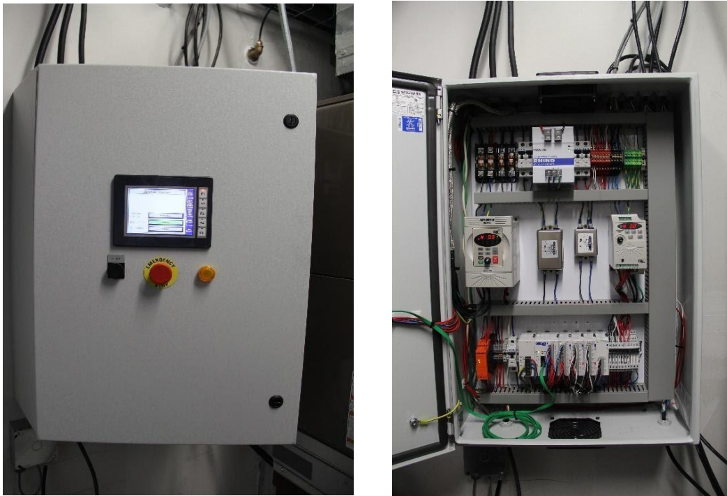
Figure 2.12: The control panel and the PLC.
