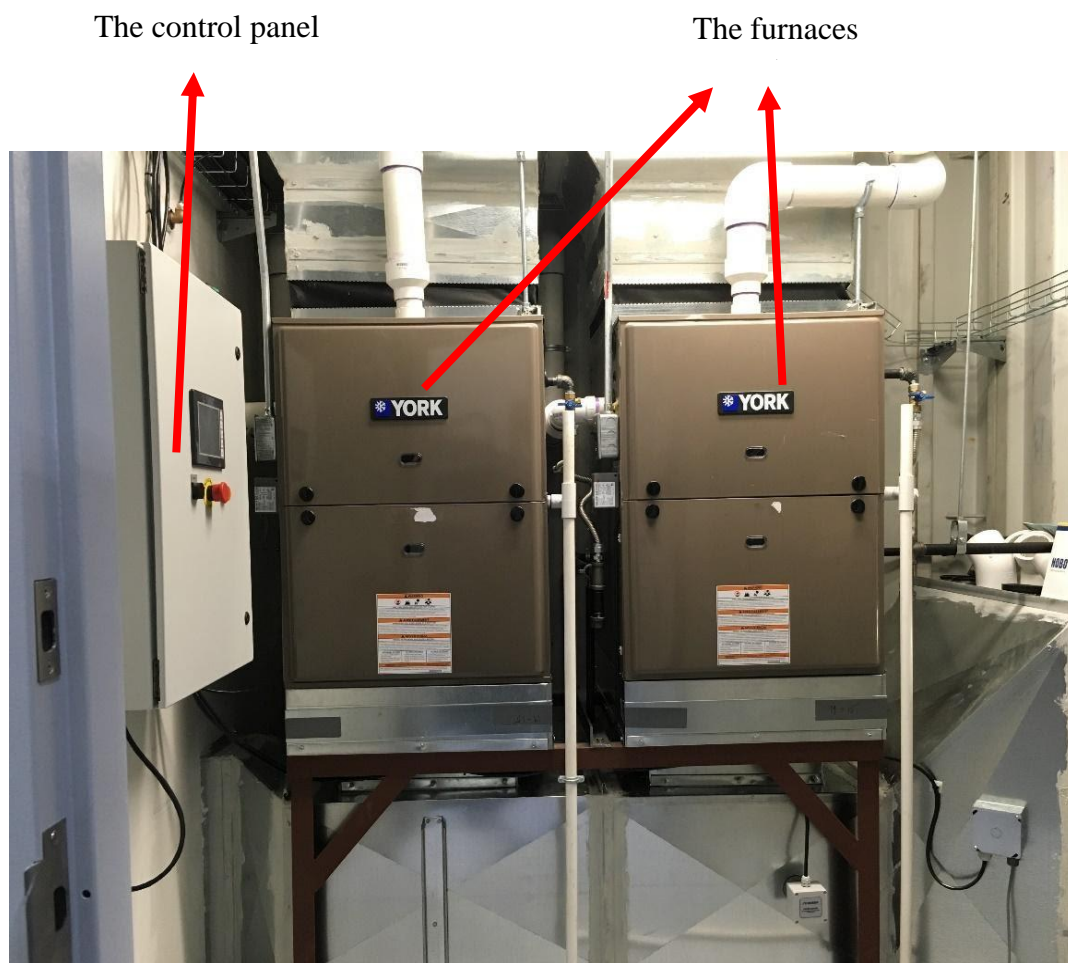
Figure 2.7: The control panel and the heaters in the control room.
