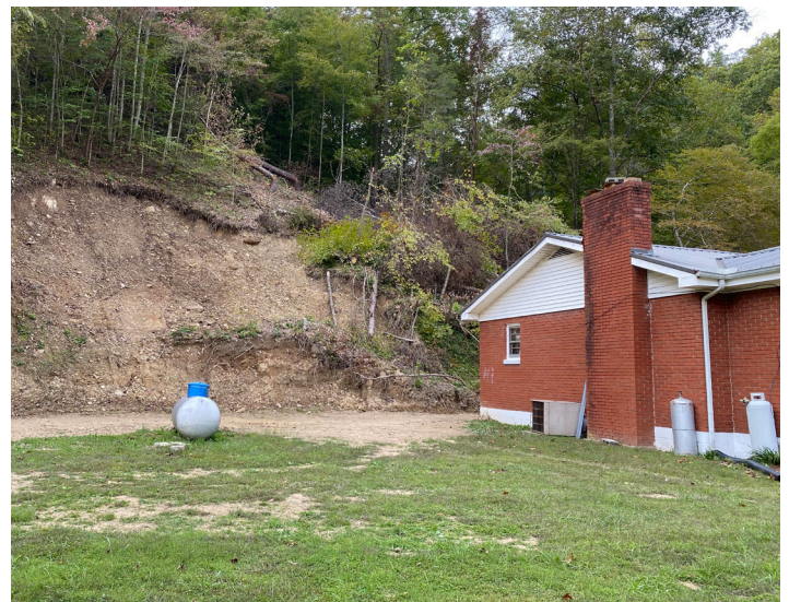
Figure 33. Translational landslide behind home near KY 28 in Breathitt County.
