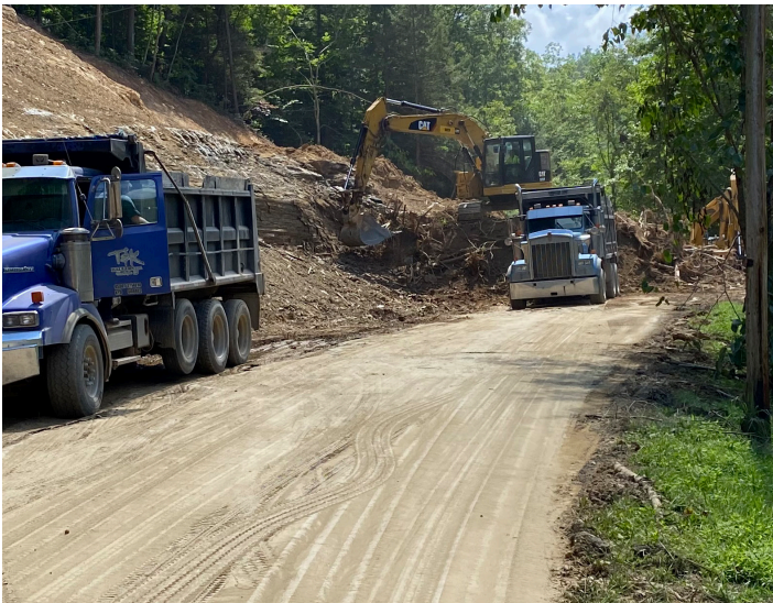
Figure 30. Trucks hauling away landslide debris along KY 267 in Perry County. The road was closed for several weeks.
