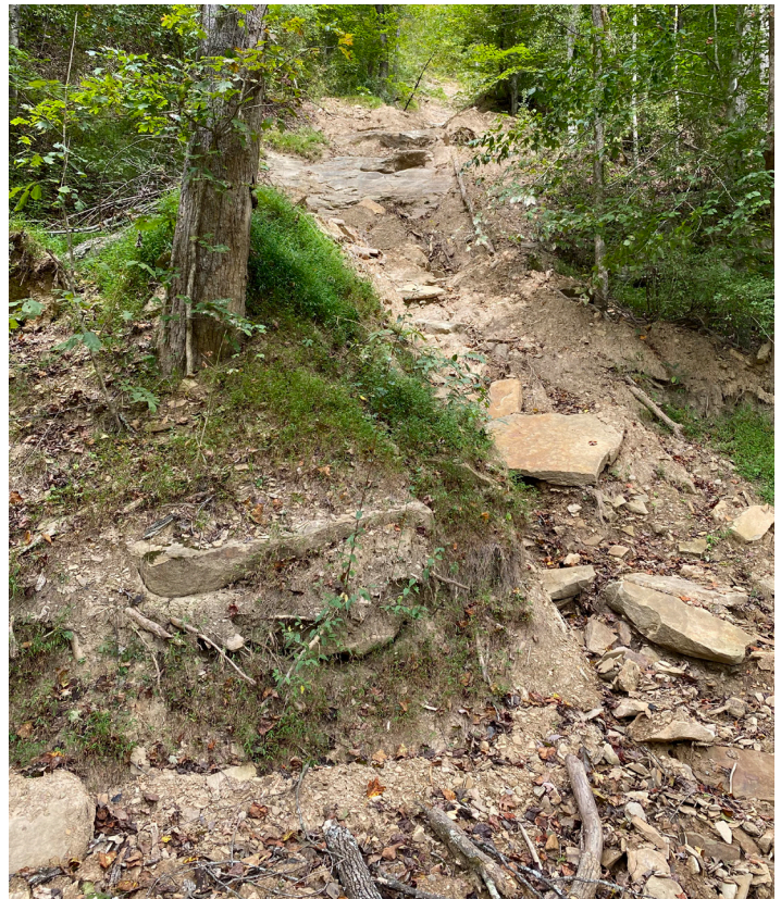
Figure 25. Narrow debris flow channel and fan deposit toward the mouth of channel along Middle Fork River Road in Perry County.
