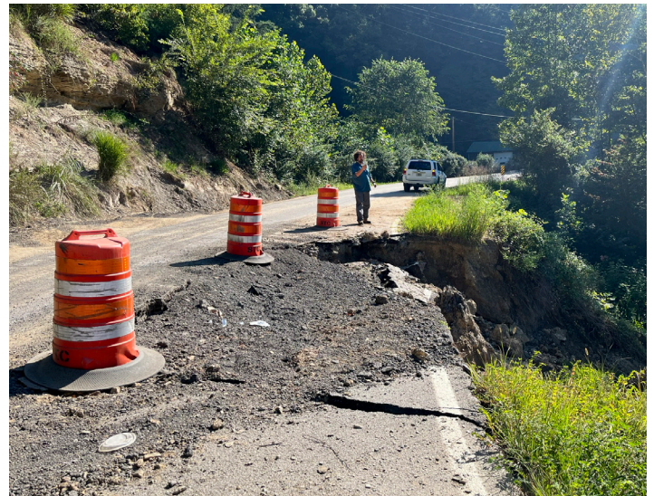
Figure 31. Landslide-damaged road along KY 2446 in Perry County.
