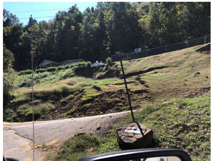
Figure 23. Slump observed off 451 in Perry County. Note the thick soil and bulging toe along the road.
