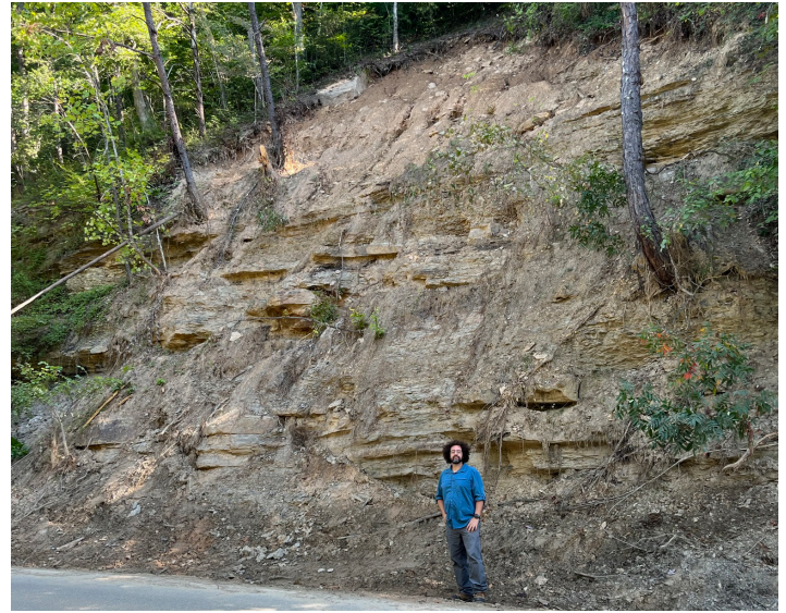
Figure 20. Photo of translational landslide along KY 2446 in Perry County, triggered by the July storms.
