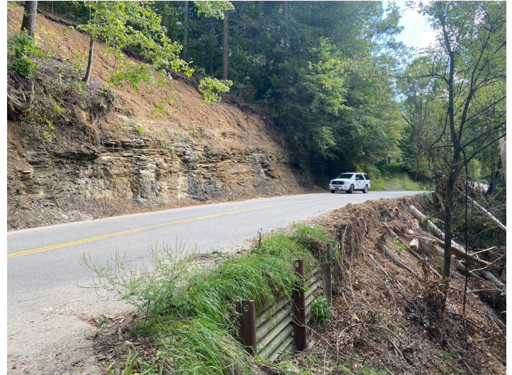
Figure 21. Photo of translational landslide along KY 28 in Perry County, triggered by the July storms
