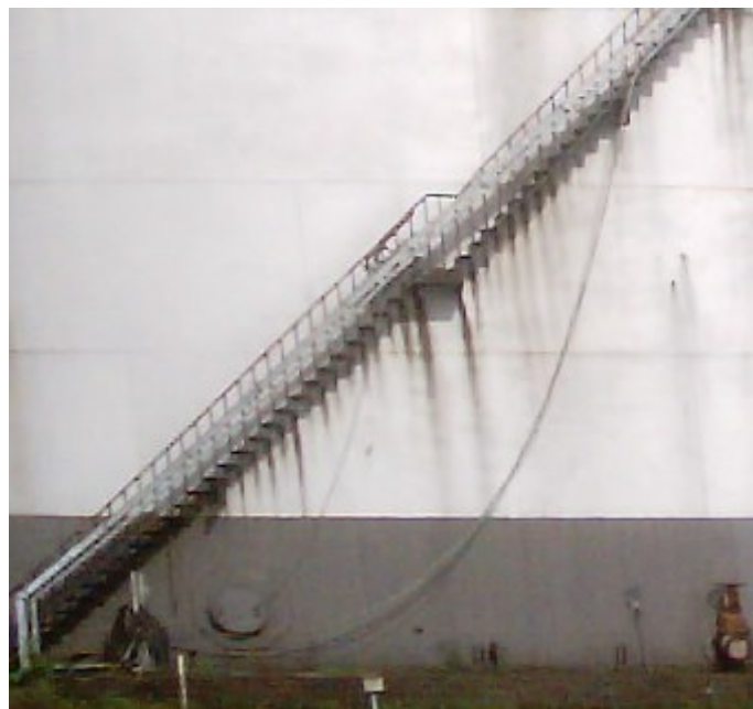
Figure 7.7. Cables dangling on the FRT's stairway
