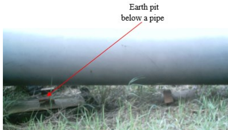
Figure 7.5. Improper grounding pit location
