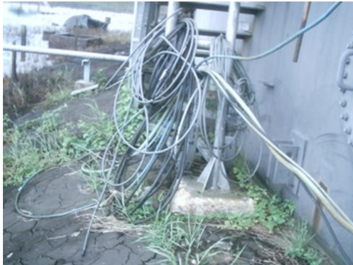
Figure 7.6. Sprawled cables around the tank shell
