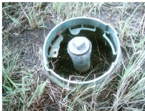
Figure 2.5. Chemically activated grounding electrode (CAGE)
