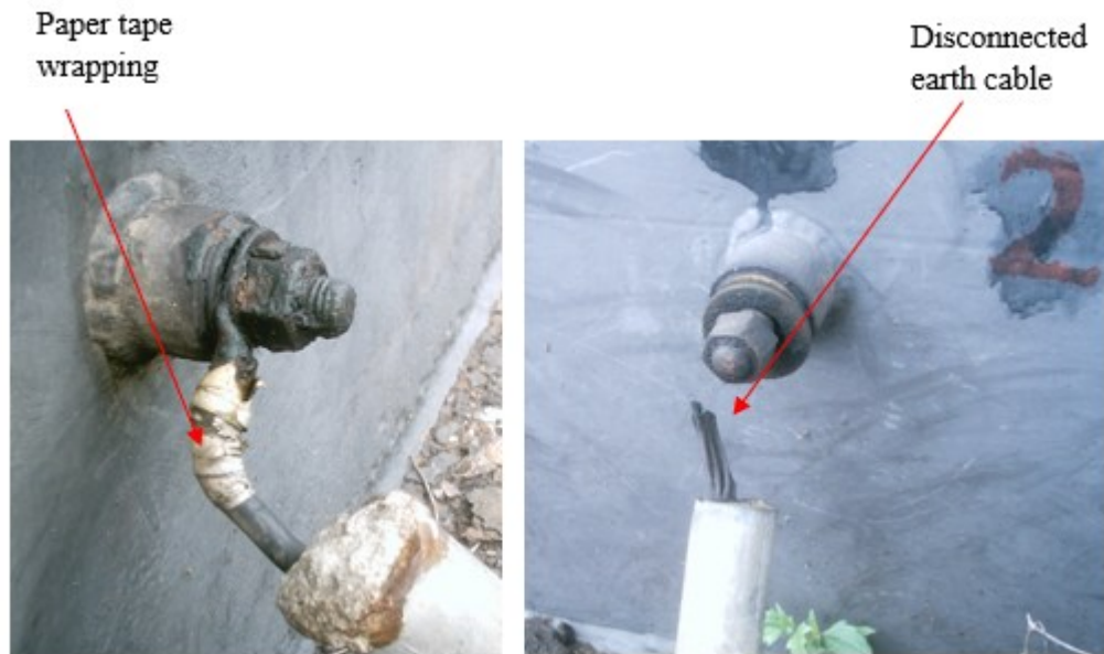
Figure 7.4. Poor grounding cable management
