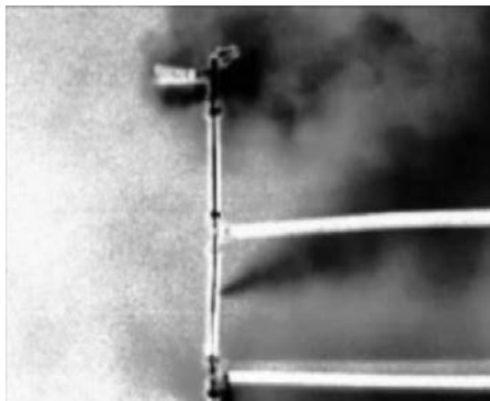
Figure 13. Two small leaks detected at a \text{CO}_2 duct with an active measurement configuration
