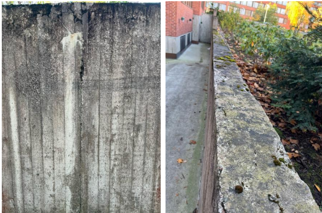
Figure 37- Visual detail of cracks and environmental effects on reinforced concrete retaining wall
