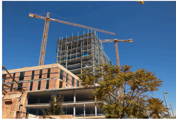
Fig. 6. The Student Hotel under construction next to the green corridor on Cristóbal de Moura. (Source: Authors, 2021)
