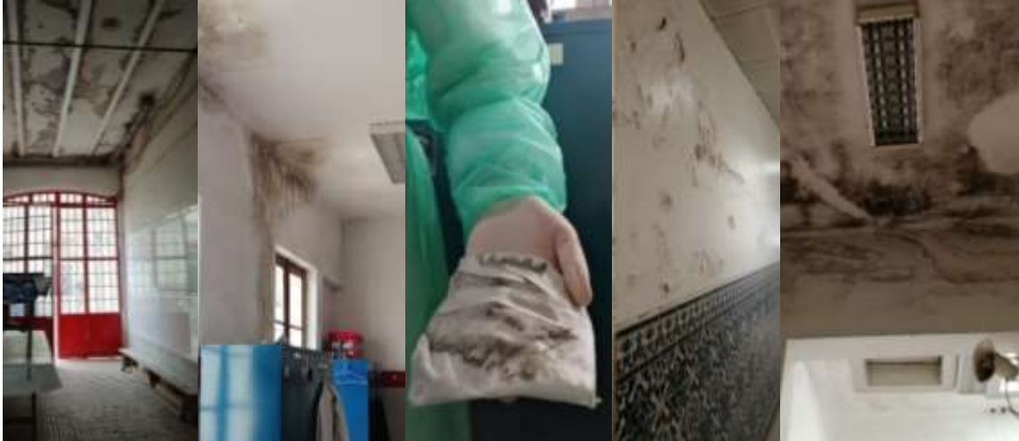
Figure 6.1- Firefighters headquarters visible problems registered during the sampling campaign.
