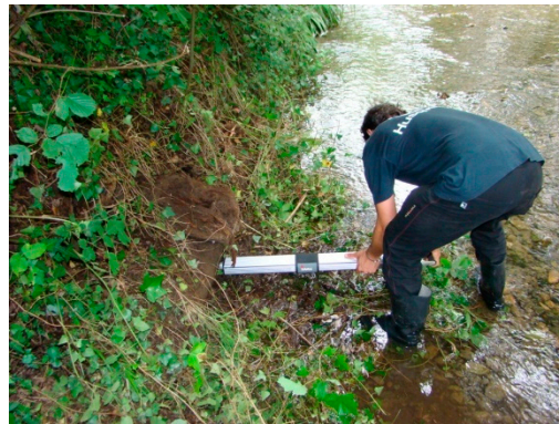
Figure 5. Analysis, by means of a resistograph, of wood deterioration processes in a log crib wall (Artia river, Irún, Guipúzcoa, Spain). Source: Guillermo Tardio.
