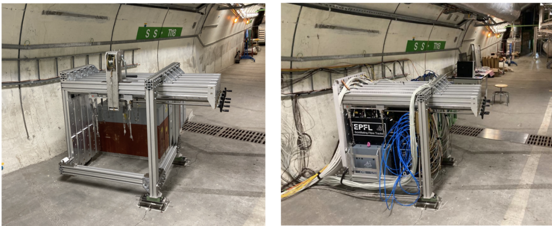
Figure 9: Mechanical support of the target system after the installation (left) and fully loaded with wall boxes and SciFi planes (right).
