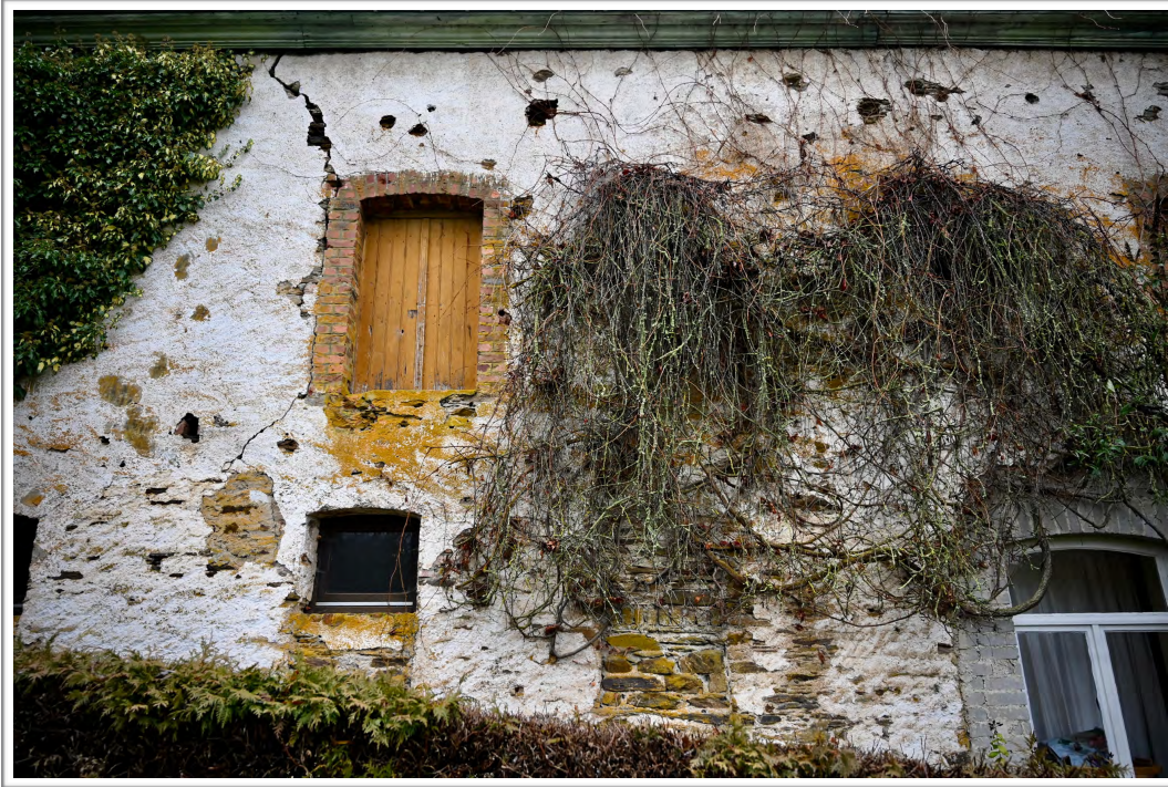
Image 1.16 Seventy-five years later, buildings in the Ardennes still bear the scars of war. This mortar-damaged building in the village of Berlé is a reminder of the dark history that many villagers remember to this day. On January 9, 1945, Berlé was liberated by the American 90th Infantry Division.
