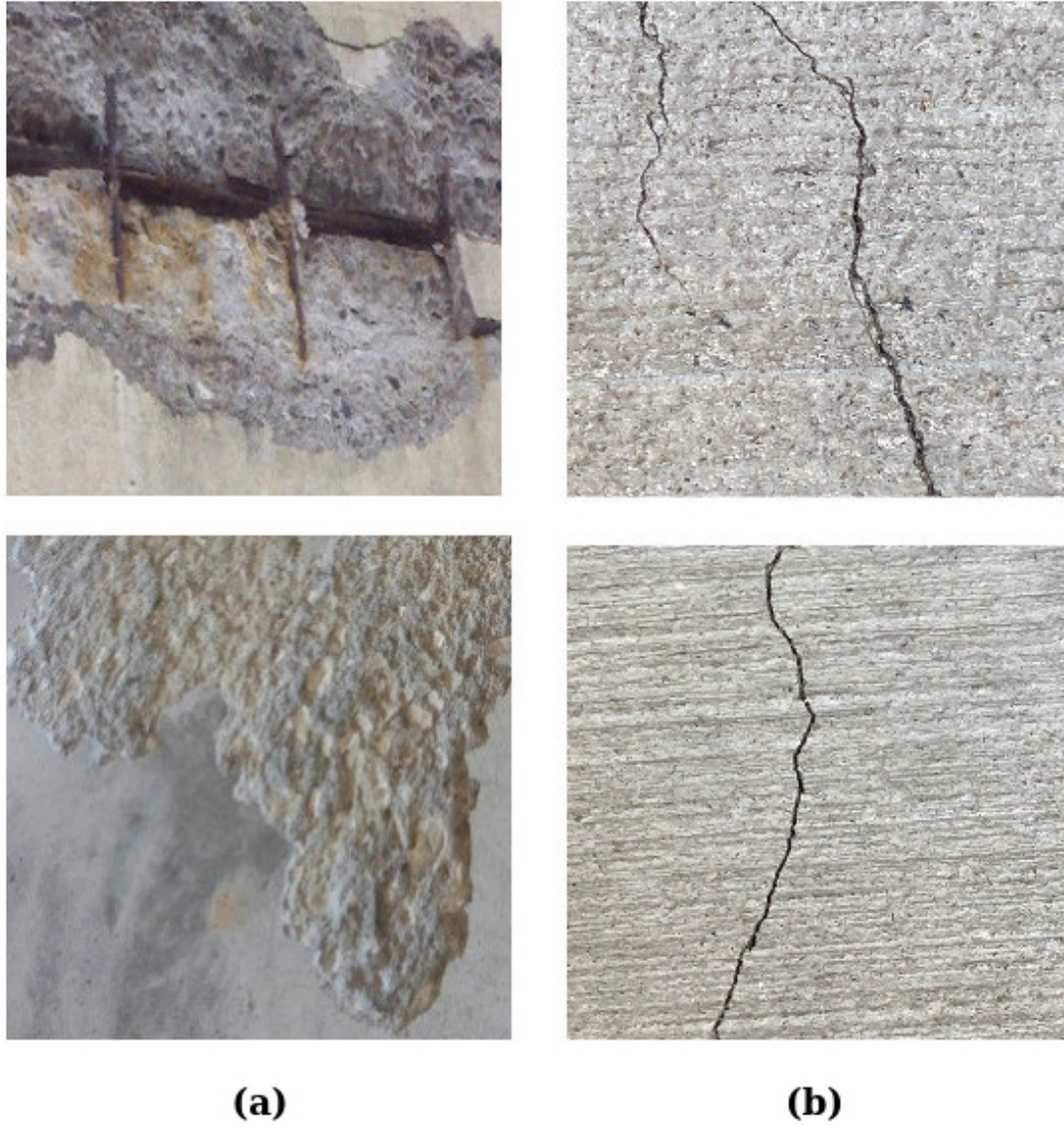
Figure 1.1: Distress in concrete: (a) Spalling (b) Cracking
