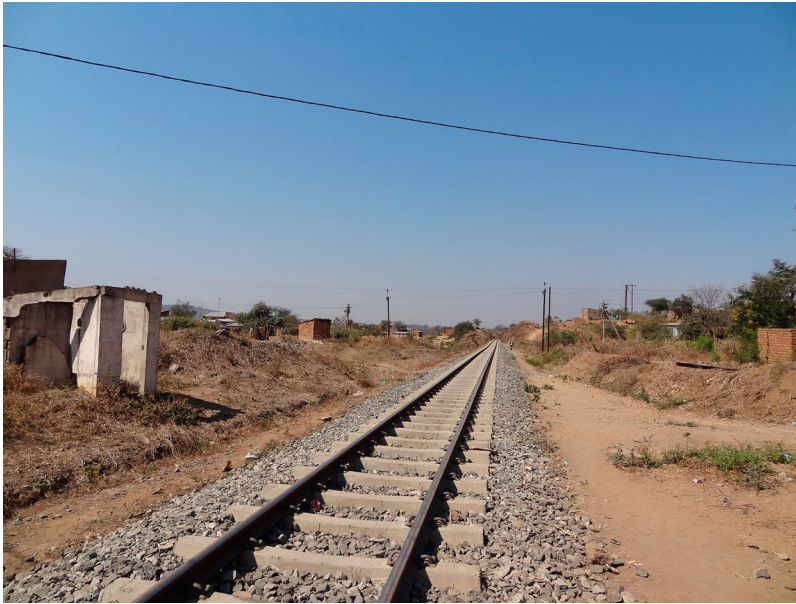
Figure 3. Railway link near Moatize mine, Tete province, in the Beira Corridor (photo by J. Kirshner).
