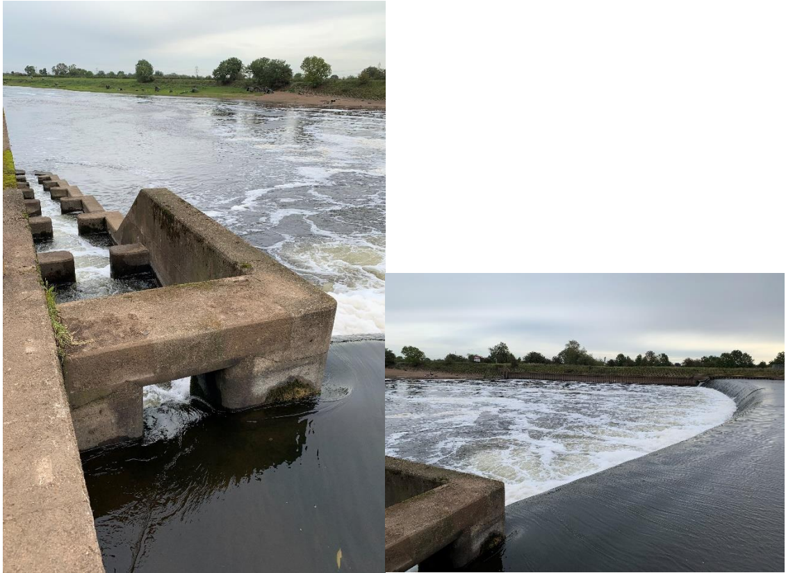
Figure 3.5. The pool and weir fish pass located at Cromwell Weir (left) and the location of the fish pass in relation to the whole weir face (right).
