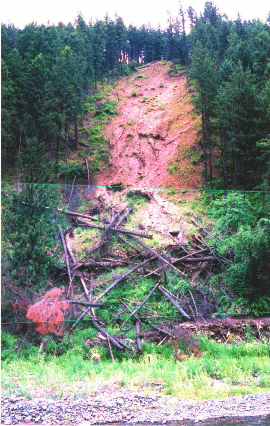
Figure 18: Photograph of Landslide at site 32. Notice pile of mixed debris at bottom of slope.
