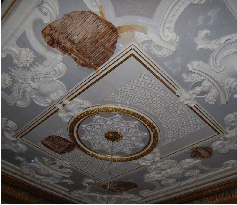
Figure 1.18: Clandon Park, the Speakers' Parlour ceiling in the days after the fire, showing its remarkable survival.
