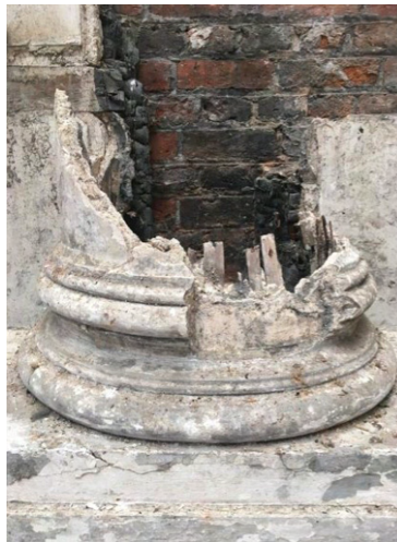
Figure 1.28: An engaged column in the Marble Hall: partially burned, it reveals the timber structure beneath the plaster.
