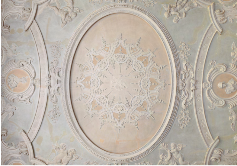
Figure 1.12: Clandon Park, the Saloon ceiling showing the coloured paint scheme introduced by John Fowler.
