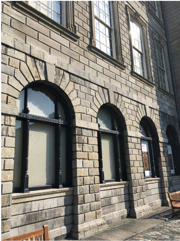
Figure 8.2: Calp limestone arcade, Old Library, Trinity College Dublin. The dark muddy limestone on the ground floor offers a visual contrast to the paler granite of the upper storeys.
