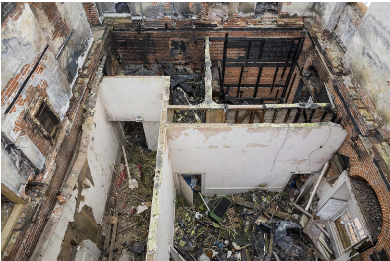
Figure 6.6: Clandon Park, Surrey, looking down into the burned-out rooms.
