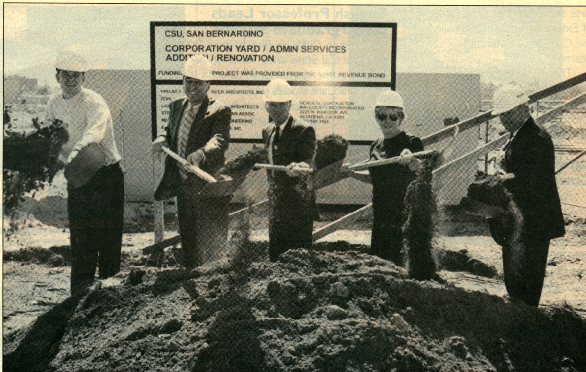
DIGGING IT —Construction and renovation of facilities housing several business administrative services at Cal State is underway on the northwest perimeter of campus. President Karnig (second from left) tosses the ceremonial dirt to start the project in October for the 50,000-gross-square-foot of renovated and expanded space that will house the Duplicating Center, receiving and mail distribution center, public safety and the maintenance shops. The new accommodations will permit the university to deliver services to an expanding campus population, now surpassing 15,000 students and employees. They replace facilities built in 1970. The project is funded by monies allocated by Proposition 203, approved by voters in 1996. Construction is expected to be completed in January, 2000.
