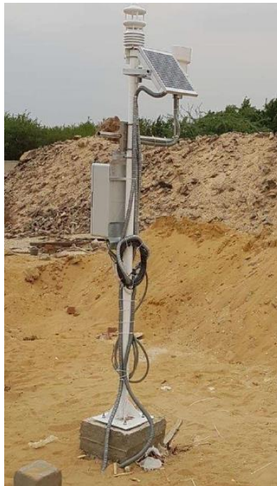
Figure 55 Installed weather station
