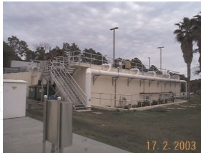
Figure 7. Septage tank with a gas buster unit installed (with TRIO 3 permitted authorization).
