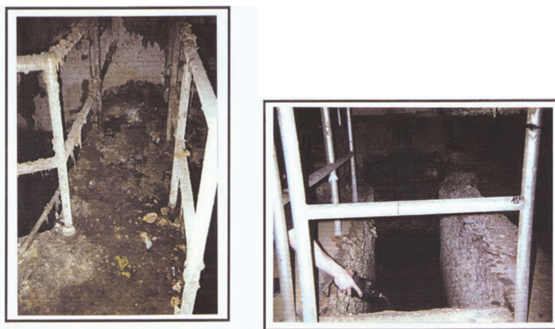
Figure 4-10. PS No. 346. Effects of Corrosion
