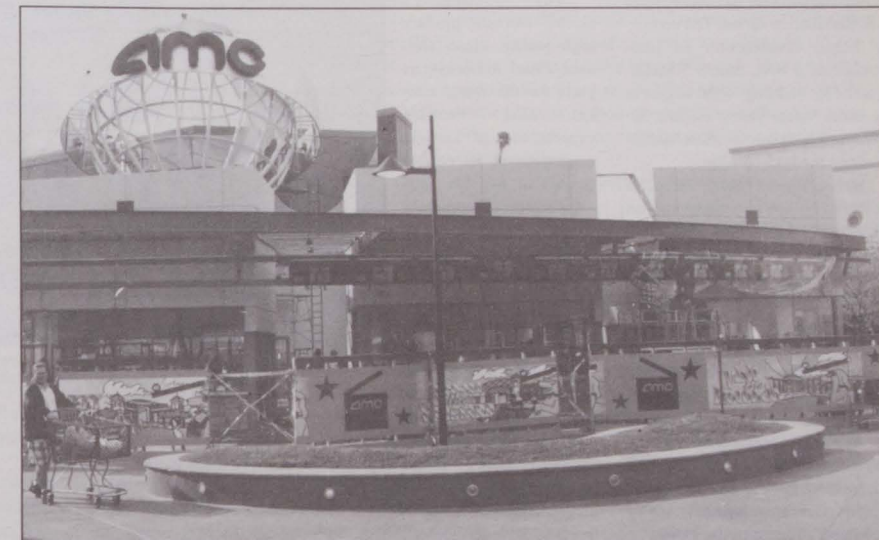
Final construction on the world's largest multiplex cinema theater, Ontario's AMC 30 located at Ontario Mills.
