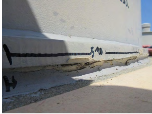
8. Cell 5 Caulking As-Found
