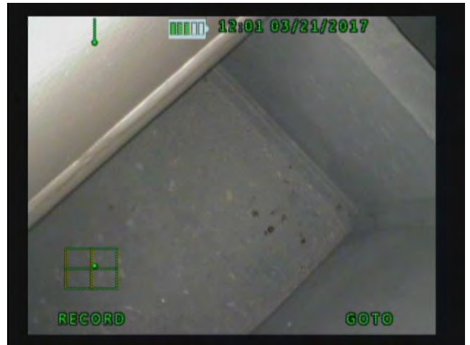
6. Vault Liner Bottom and Seismic Shim
