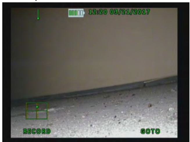
12. Overpack and Vault Liner Bottom with Debris
