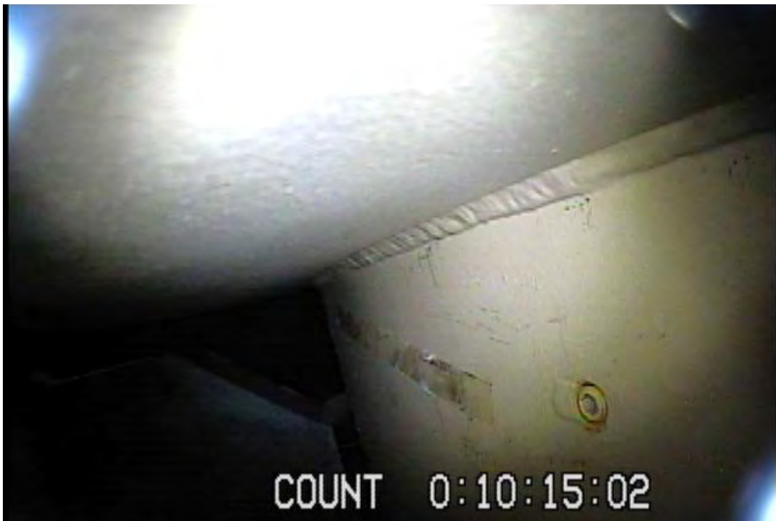
43. Overpack south east section (light rust around set screw)
