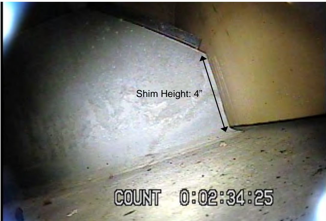
41. Overpack north section coating scrape adjacent to seismic shim
