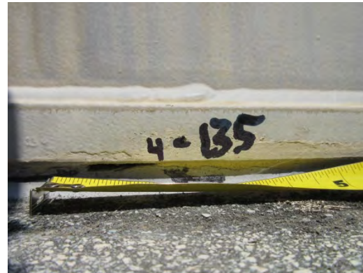
6. Cell 4 Caulking As-Found
