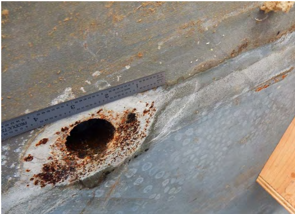
8. Underside hole #5 showing corrosion prior to cleaning
