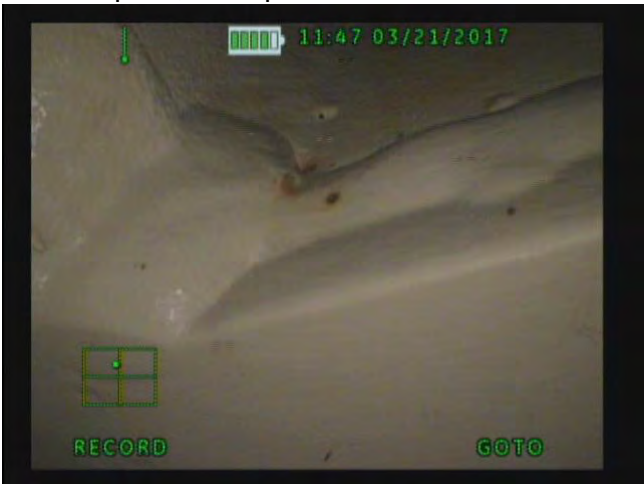
21. Overpack, rust spots
