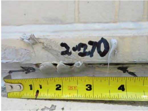
3. Cell 2 Caulking As-Found
