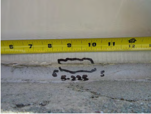
13. Cell 5 Caulking As-Found
