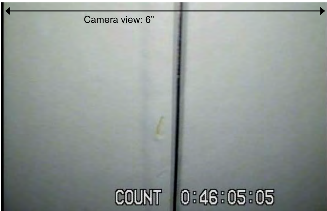
27. Scan 26 coating chip with slight rust discoloration
