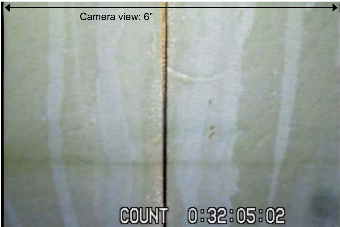
61. Scan 76 rust spots
