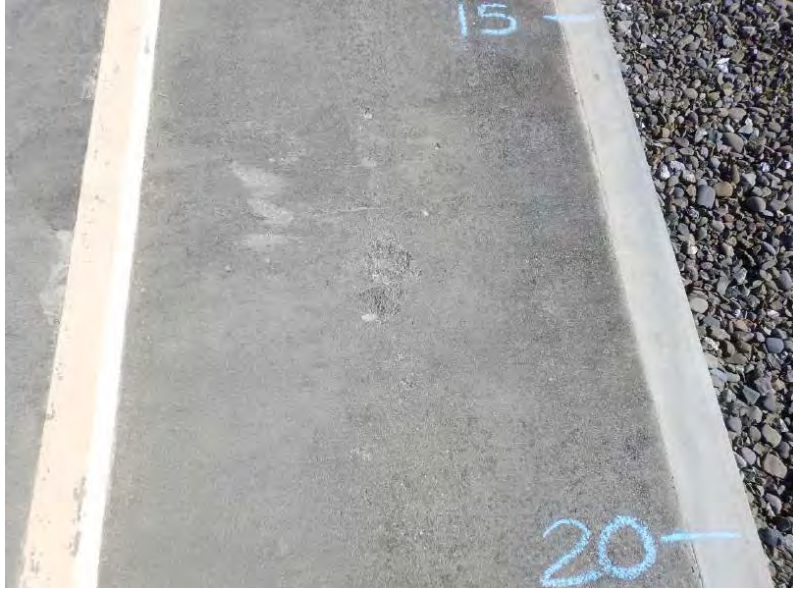
1. South side surface scaling/peeling at (18, 17) that is approximately 5" wide by 10" long by 3/8" deep
