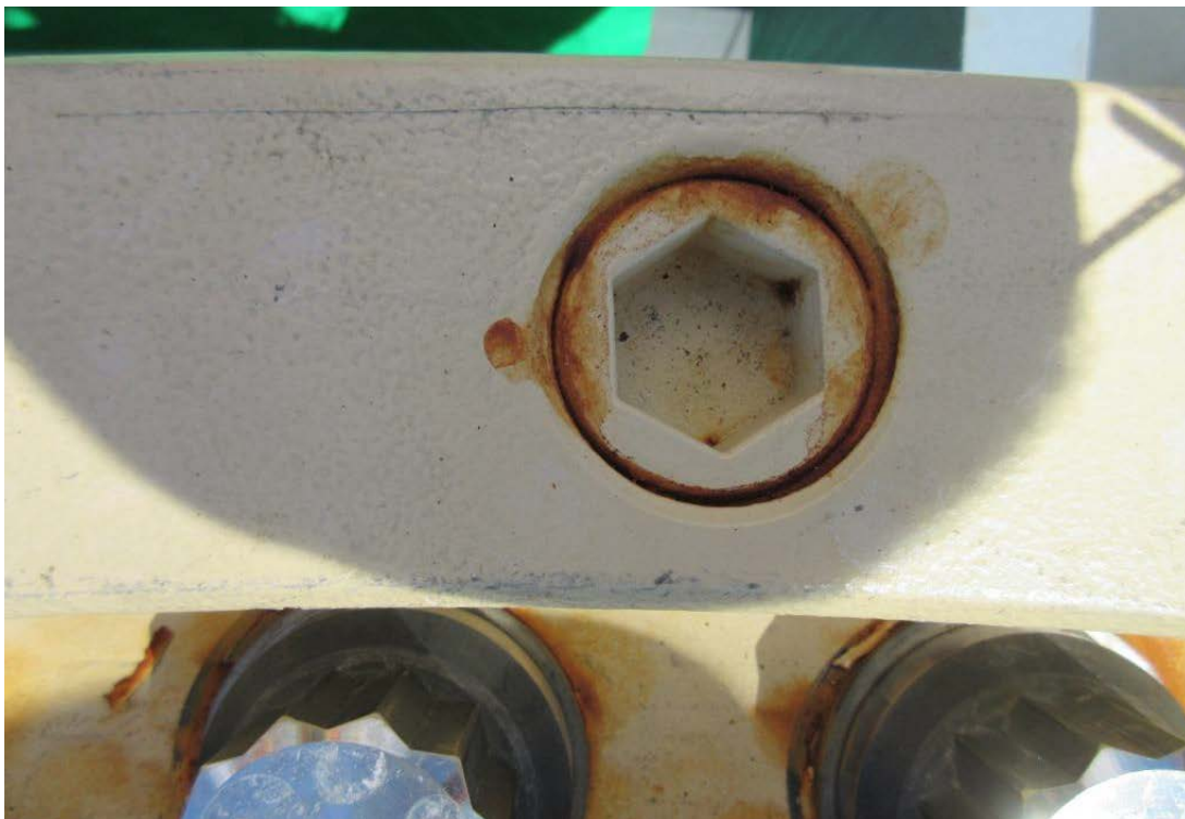
18. Typical rust staining around top flange closure plug set screws
