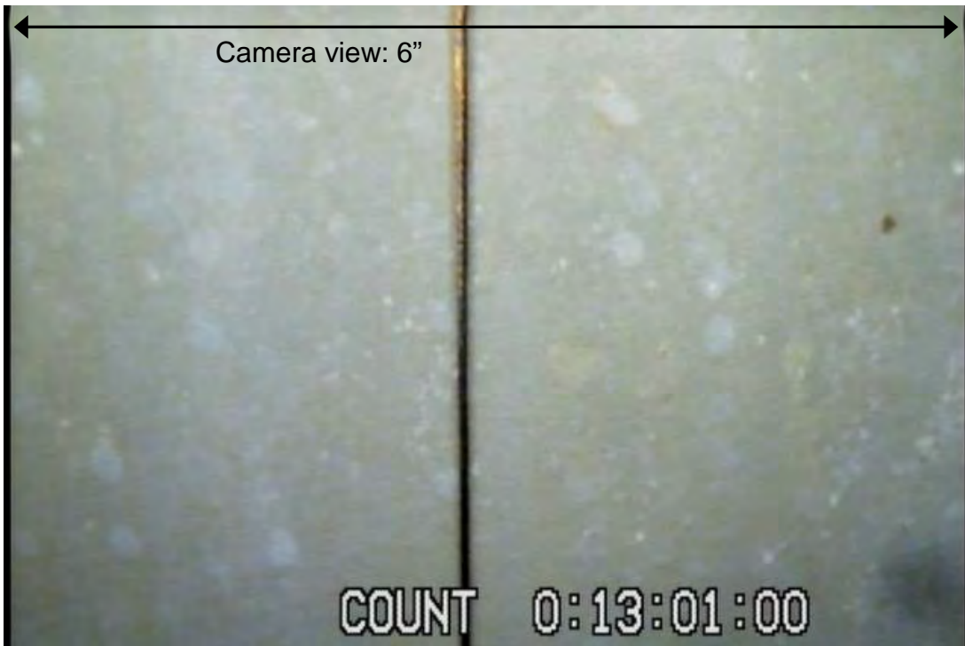
57. Scan 8 rust spot
