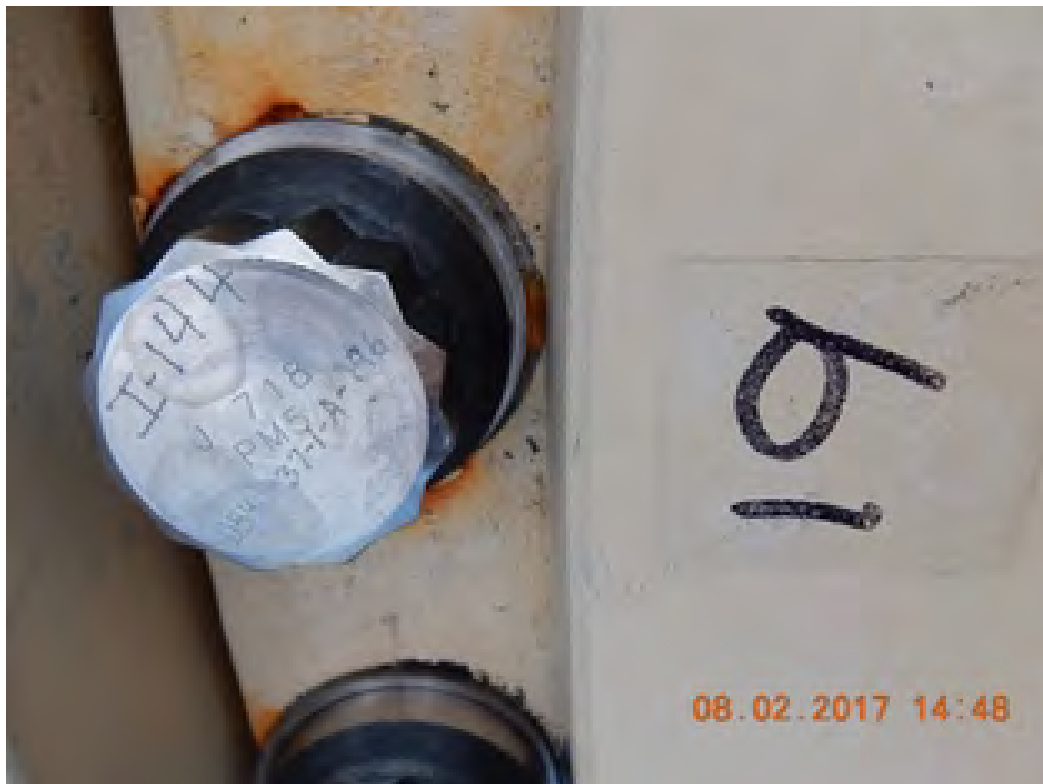
20. Cracked coating under overpack closure lid bolt
