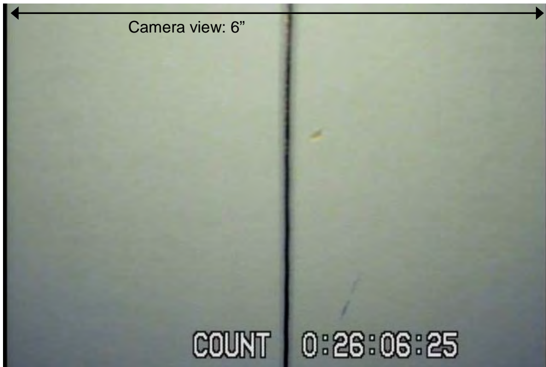
35. Scan 55 slight rust discoloration
