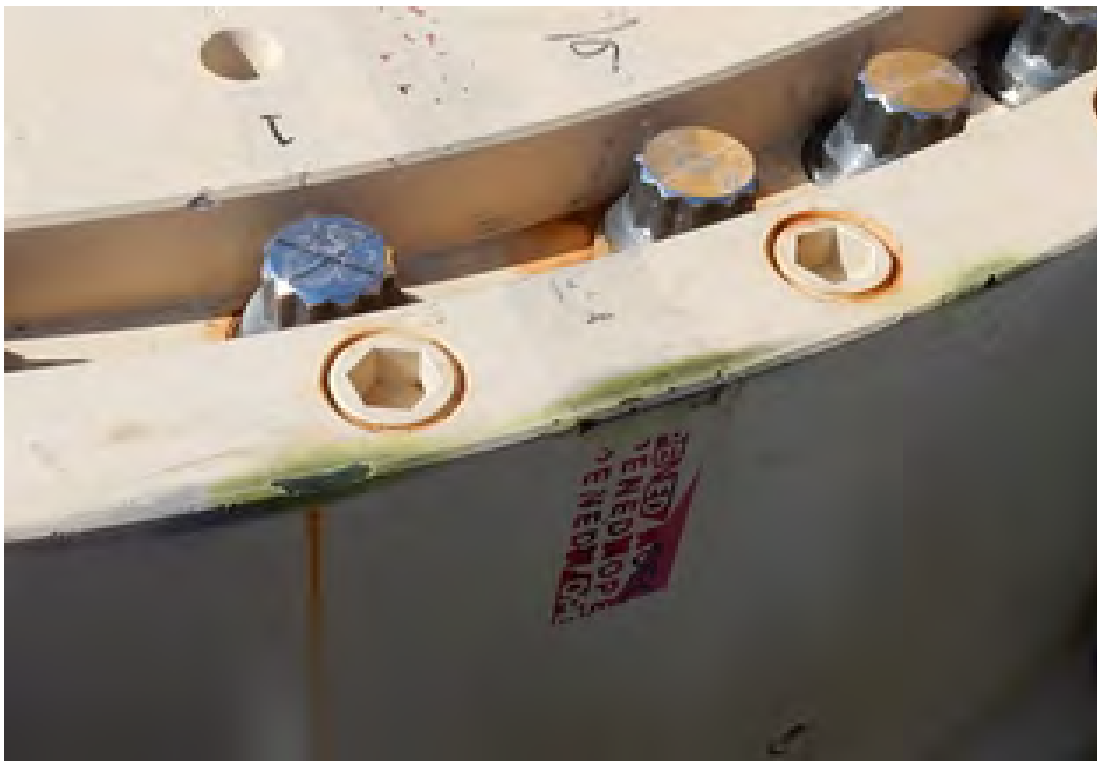
22. Coating chip from photo 21 (next above) after Rustbond epoxy sealer repair
