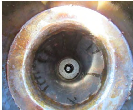
64. Inside lid bolting access hole evidence of moisture intrusion
