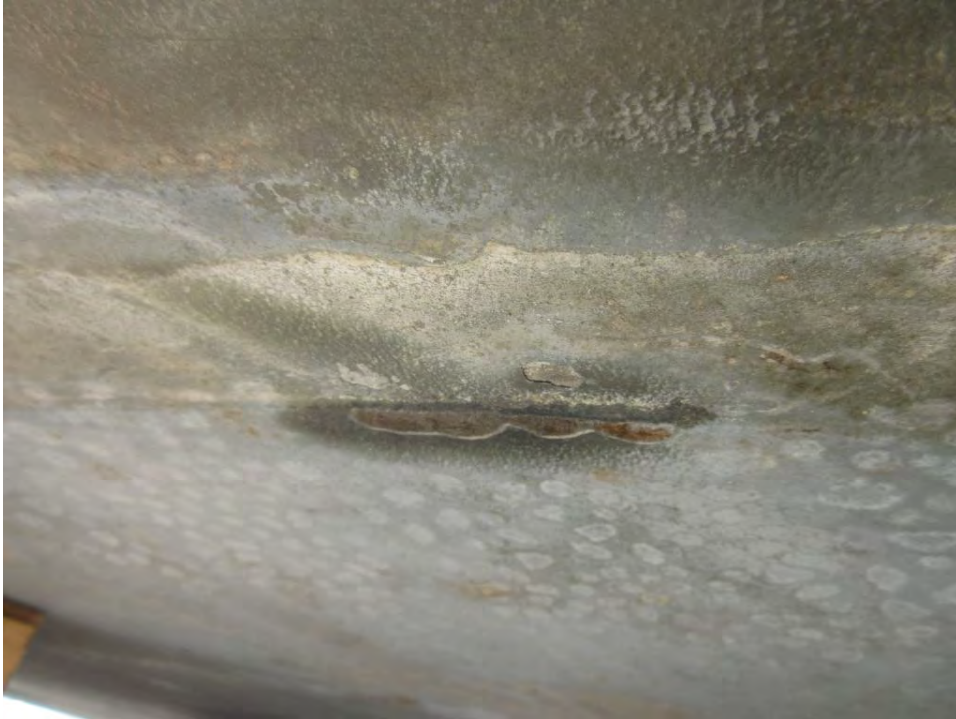
13. Coating chip on underside of lid
