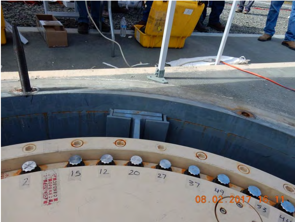
50. Rust staining at vault lid ring to vault liner interface
