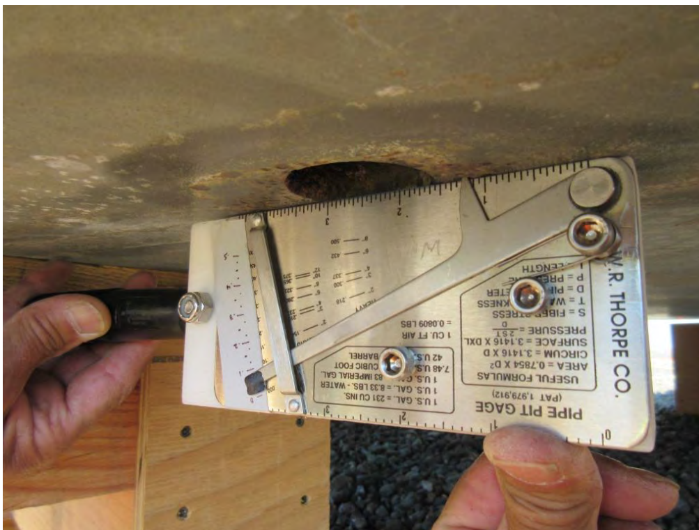
12. Measuring pit depth <math><1/16''</math>
