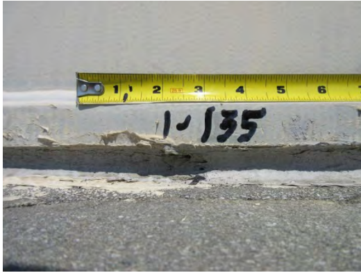
1. Cell 1 Caulking As-Found
