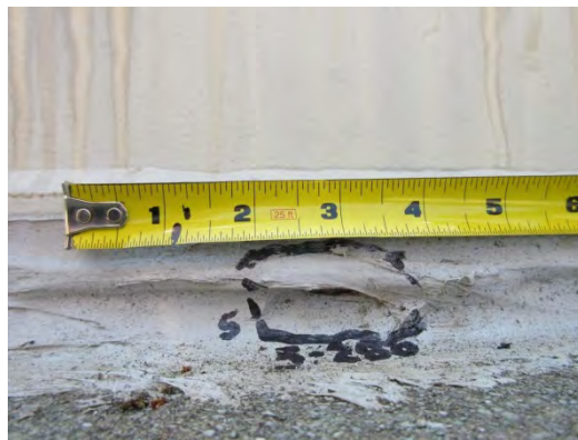
12. Cell 5 Caulking As-Found
