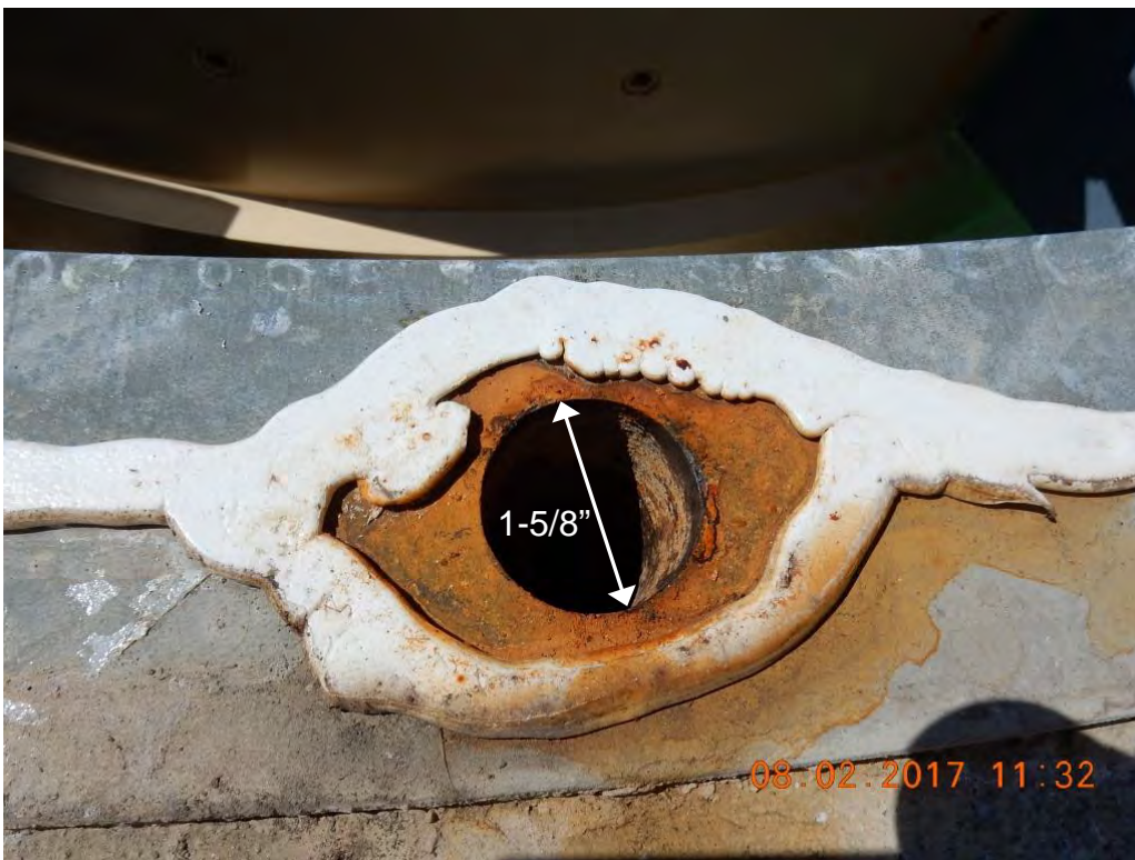
47. Vault lid ring bolt hole #6 corrosion products
