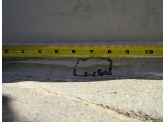
14. Cell 5 Caulking As-Found
