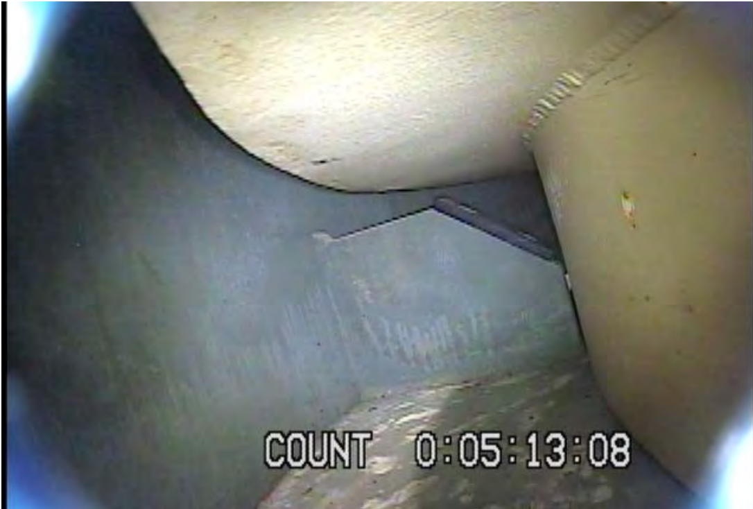
40. Overpack underside northeast section coating chip
