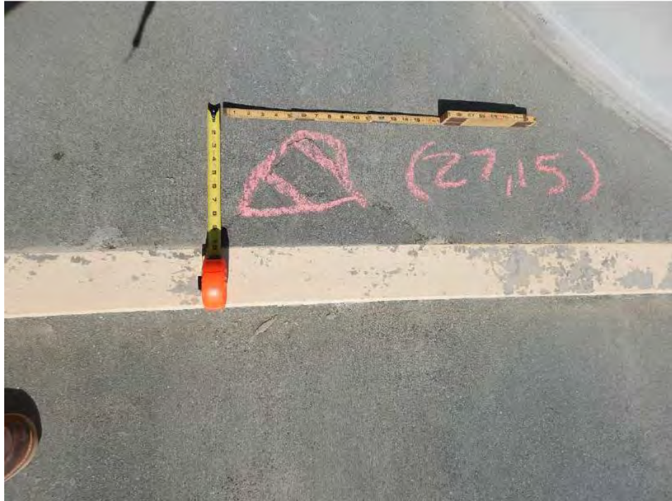
3. Center disbanded patch at (27, 15) that is approximately 8" by 6"
