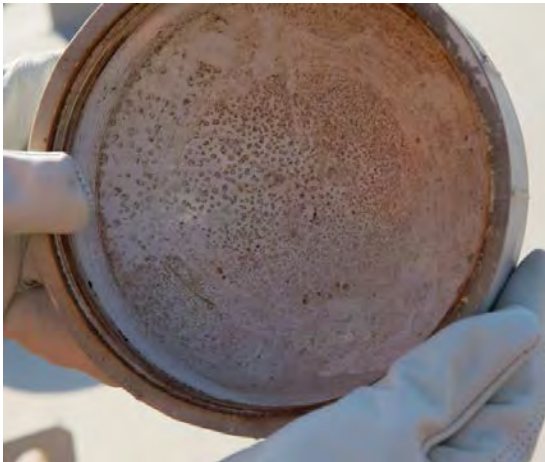
63. Underside of bolting pipe cap showing evidence of condensation
