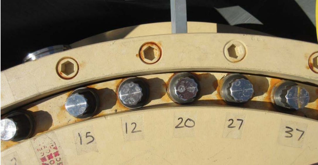
16. Rust staining around overpack lid closure bolting and around top flange plug set screws
