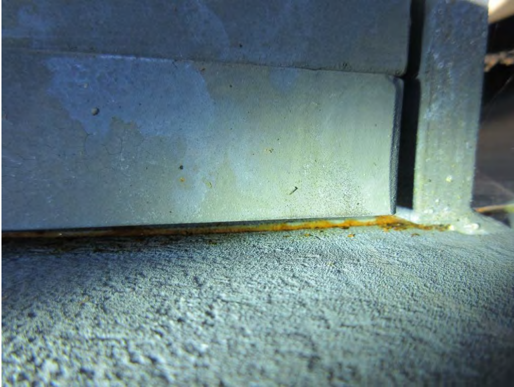
52. Rust staining at vault lid ring to vault liner interface (view looking down along liner with seismic shim in upper portion of the picture)
