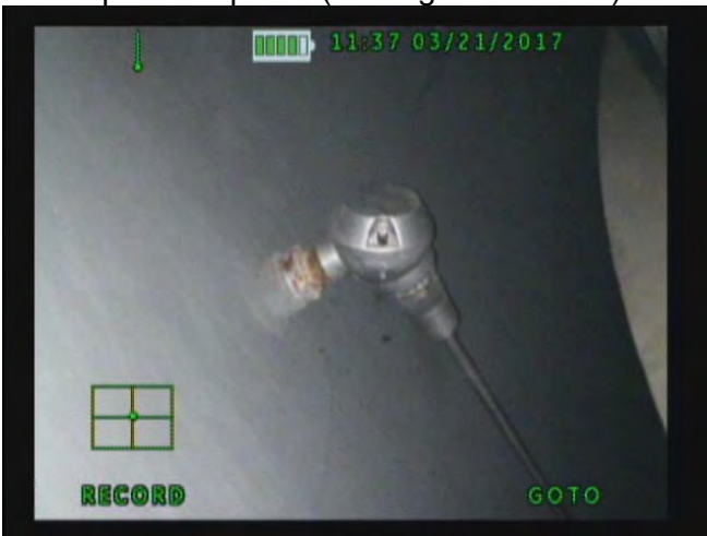
3. Temperature probe (no longer in-service)
