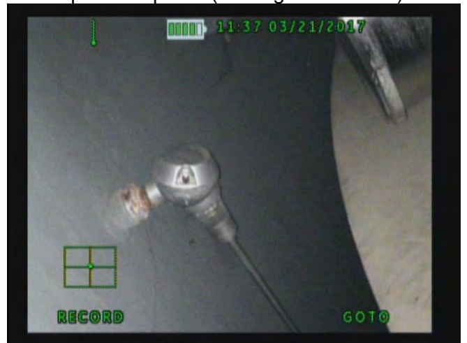
4. Temperature probe (no longer in-service)
