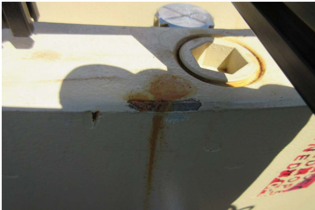
21. Coating chip with rust staining
