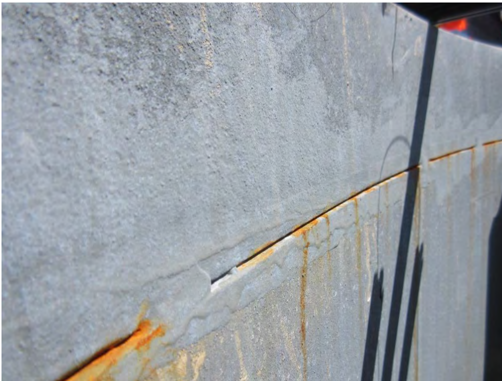
51. Rust staining at vault lid ring to vault liner interface
