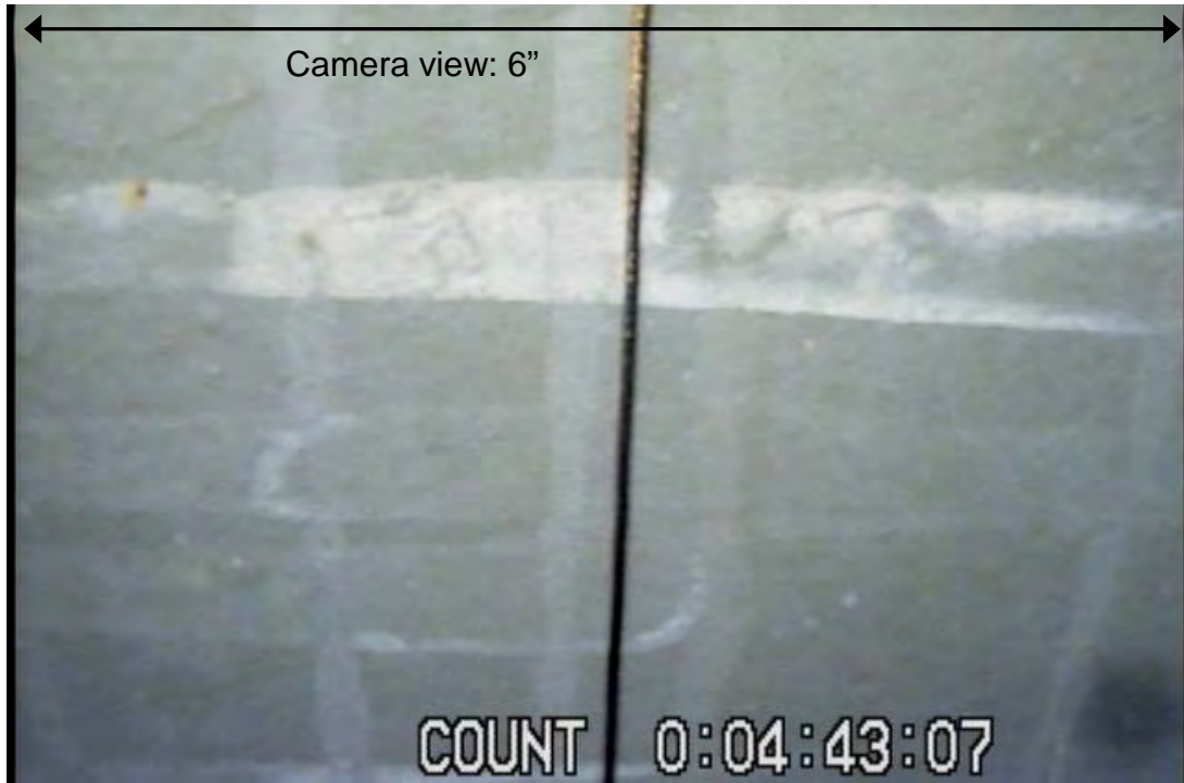
54. Scan 5 rust spot
