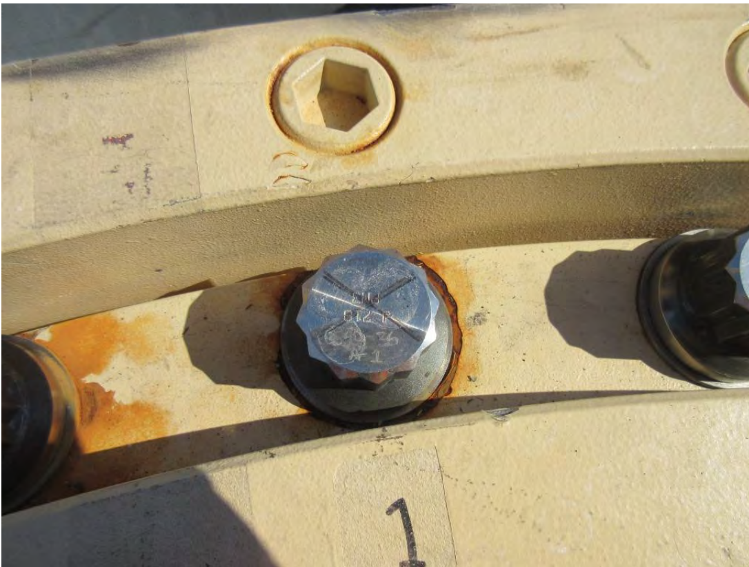
17. Rust staining around overpack lid closure bolting
