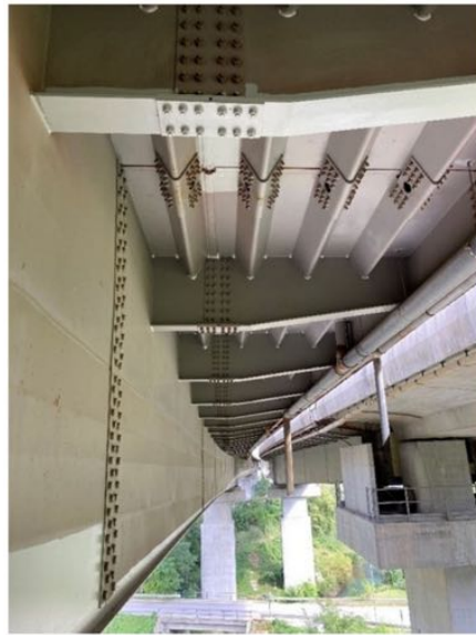
Figure 13. View of the right cantilever of the deck of the case study.
