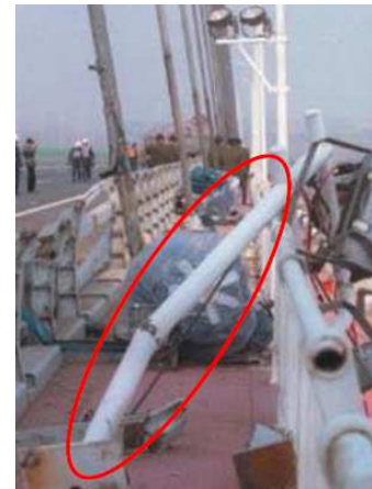
Fig 1. Cable damage in Haiyin Bridge [4].
