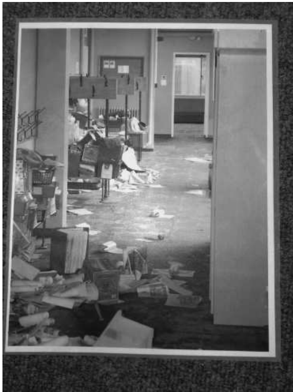
Figure 4 Damage (from Primary School notice board).
