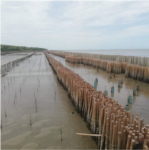
FIGURE 4 Bamboo dykes built to protect against erosion (own source)
