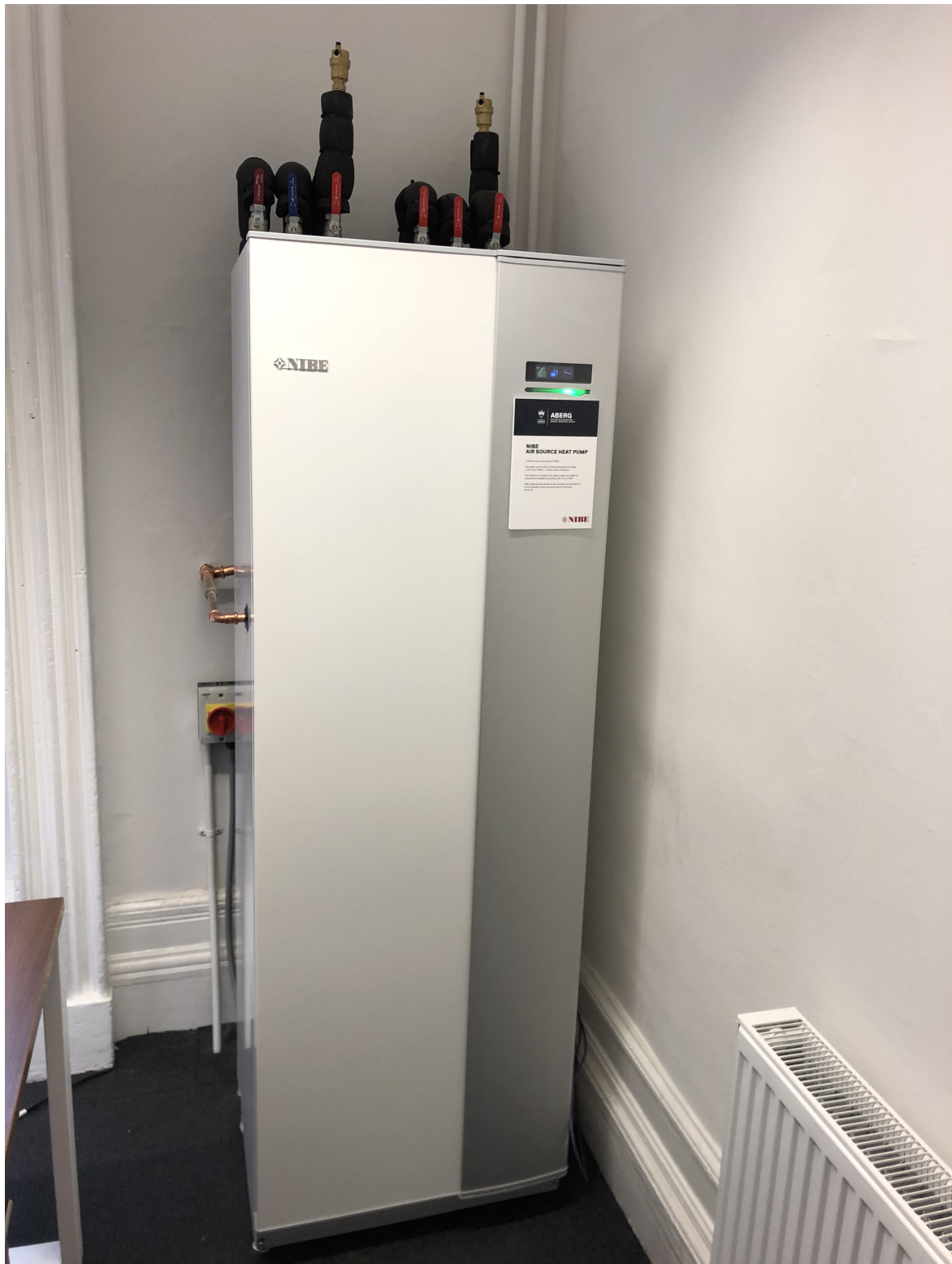
Figure 4.6: HP indoor unit at Salford Smart Meters Lab
