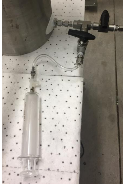
Figure 5-9 Oil sampling connection in oil sampling process
