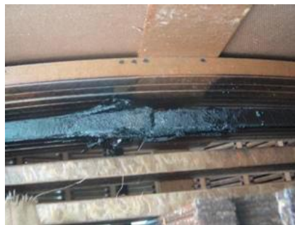
Figure 2-1 winding fault in a 400/132kV 240MVA transformer [16]
