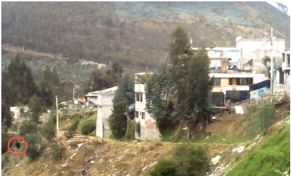
Figure 4.12. Wastewater pipe/septic tank La Roldós . Note outlet (circled in red) on ravine wall (author's photo).
