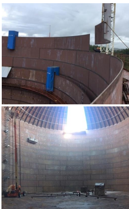
Figure 2. Appearance of the first (inner) mantle on one of the tanks, during manufacture.
