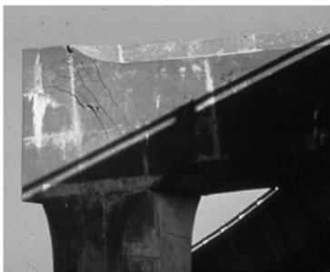
d) Pukotine na čvoru spoja greda-stub. d) Cracking of beam-column connection.
