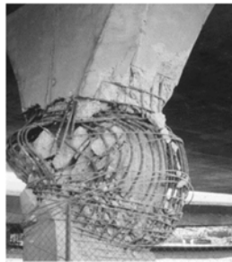
b) Slom pritisnutog utegnutoh betona, tokom loma uzengija. b) Compression failure of confined concrete.
