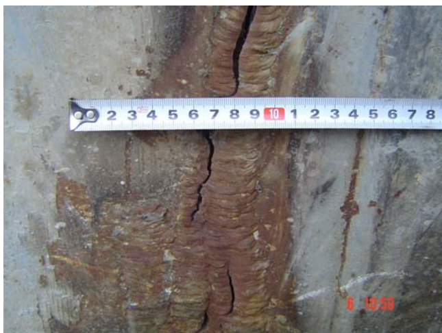
Slika 3. Pukotine na vertikalnom limu obrtne platforme (spolja) Figure 3. Cracks on vertical panel of revolving platform (outside).
