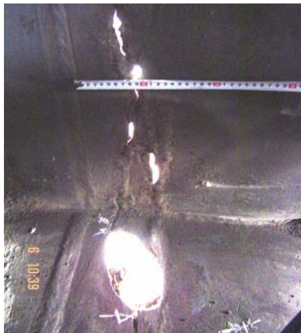
Slika 4. Pukotine na donjoj ploči i vertikalnom limu obrtne platforme (iznutra) Figure 4. Cracks on lower plate and vertical panel of revolving platform (inside).
