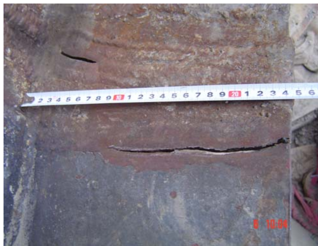
Slika 2. Pukotine na donjoj ploči obrtne platforme (spolja) Figure 2. Cracks on lower plate of revolving platform (outside).
