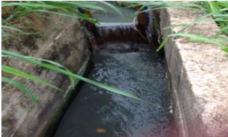
Figure 4: Wastewater Channel and Fabricated weir
