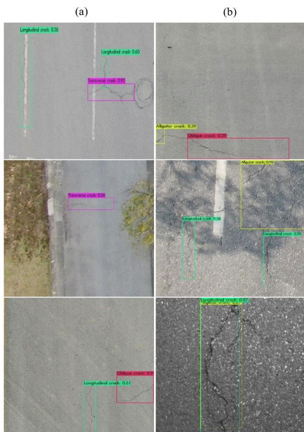
Figure 6. Some samples of the model's (a) ability and (b) inability in crack recognition.
