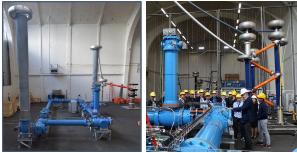
Fig. 47 Test set-up of a HVDC GIS prototype installation test.
