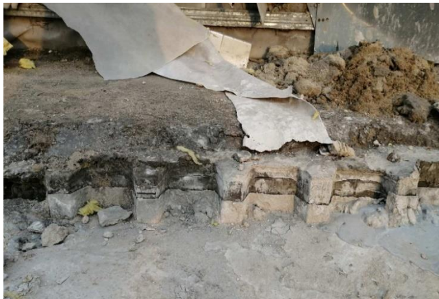
Fig. 5 The process of eliminating uneven precipitation of the foundation plate in the process of soil injection.
