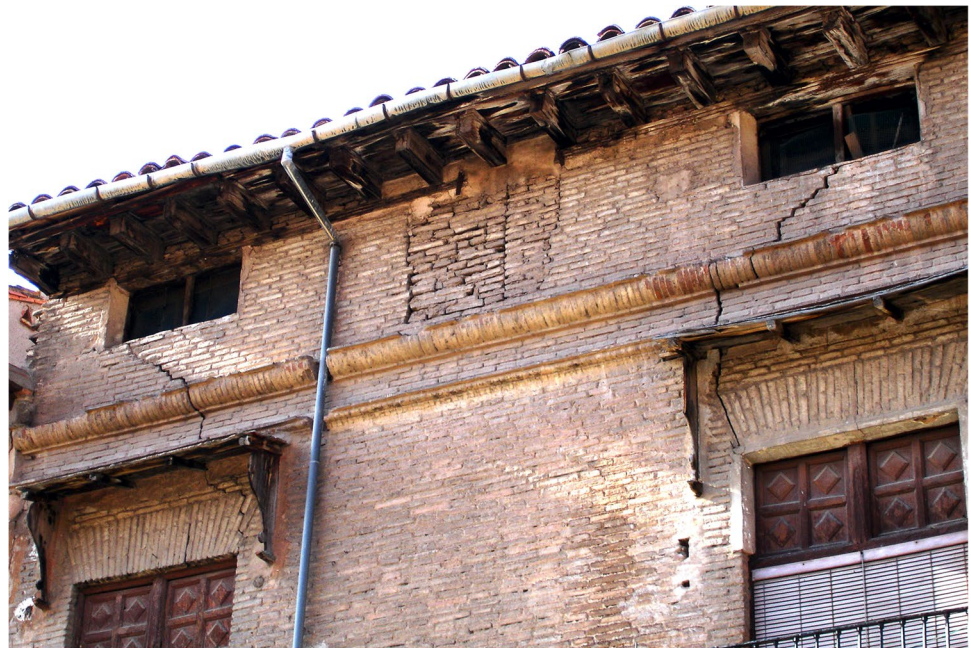
Fig. 6 Symmetrical cracks in the façade of a building in Calle Mayor of Daroca town
