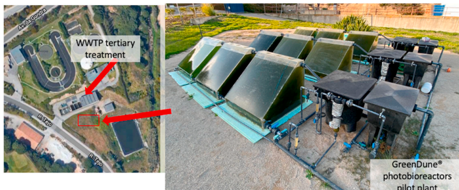
Fig. 1. GreenDune photobioreactors placed at the wastewater treatment plant of Quinta do Lago (Algarve, Portugal).
