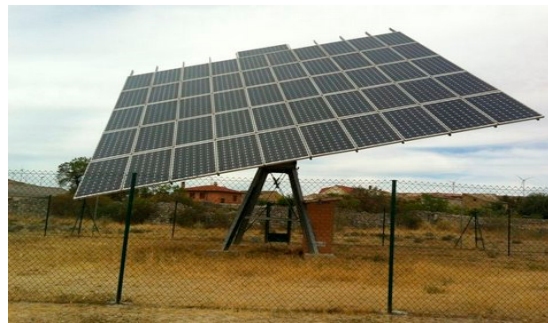
Figure 4. System 3 facility located at Los Balbases (Burgos). Two-axis sun tracker.
