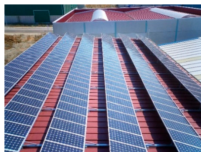
Figure 2. System 1 facility located in the city of Palencia. Fixed roof panels.
