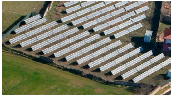
Figure 3. System 2 facility located at Torquemada (Palencia). One-axis, manual stationary tilt.
