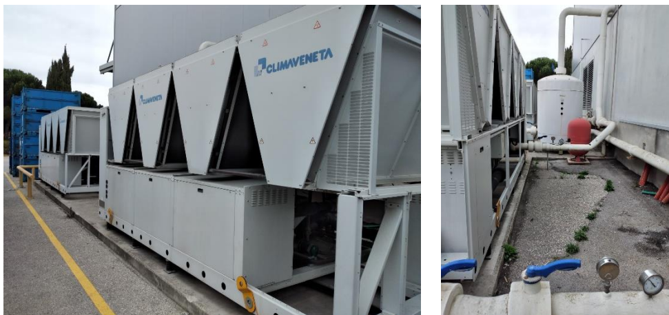
Figure 26: Cold Water Central
