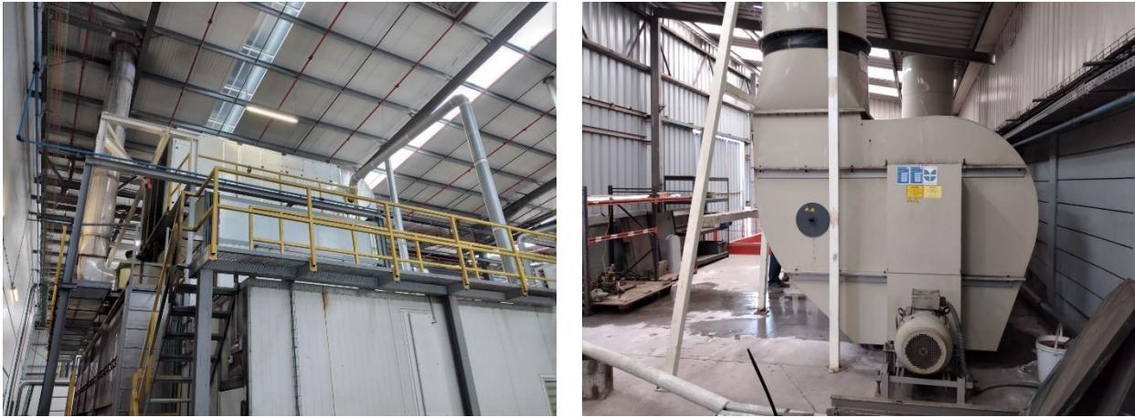
Figure 27: Ventilation equipment (L8, Scrubber L7)
