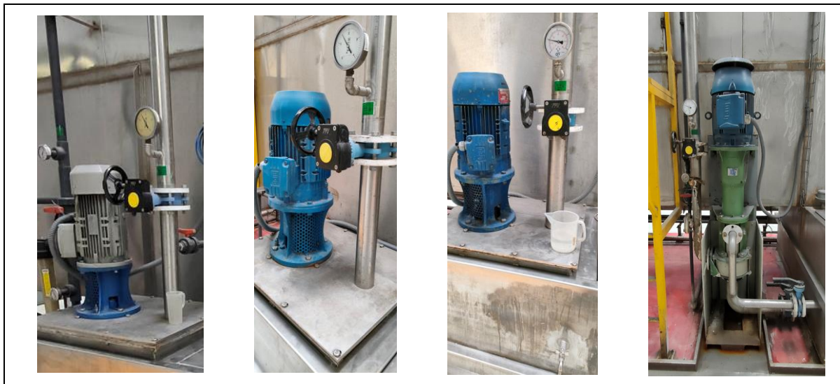
Figure 70: Line 8 tunnel pumps
