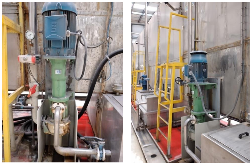
Figure 64: Line 8 shower pumps
