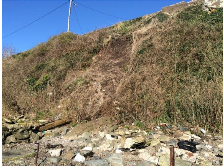
Figure 2. 4 Landslide at the Connolly Street slope prior to any preventative measures (1)
