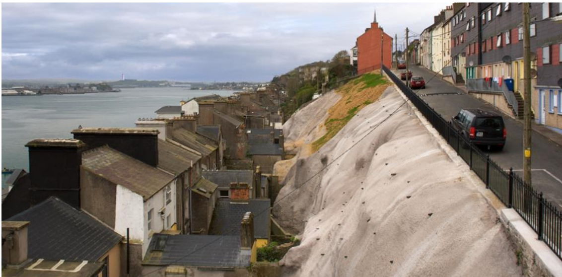
Figure 2. 2 Shotcrete protection on a slope in Harbour Row, a slope previously at risk of collapse (3)
