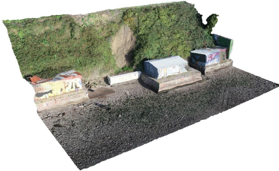
Figure 5. 9 Connolly Street slope coloured mesh
