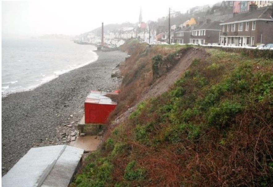
Figure 1. 1 displays the landslide on Connolly Street slope and its proximity to a primary road (1)
