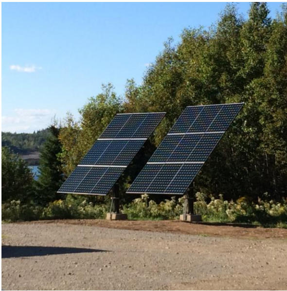
Figure 19. 6.2 kW of fixed-position solar photovoltaics facing south.
