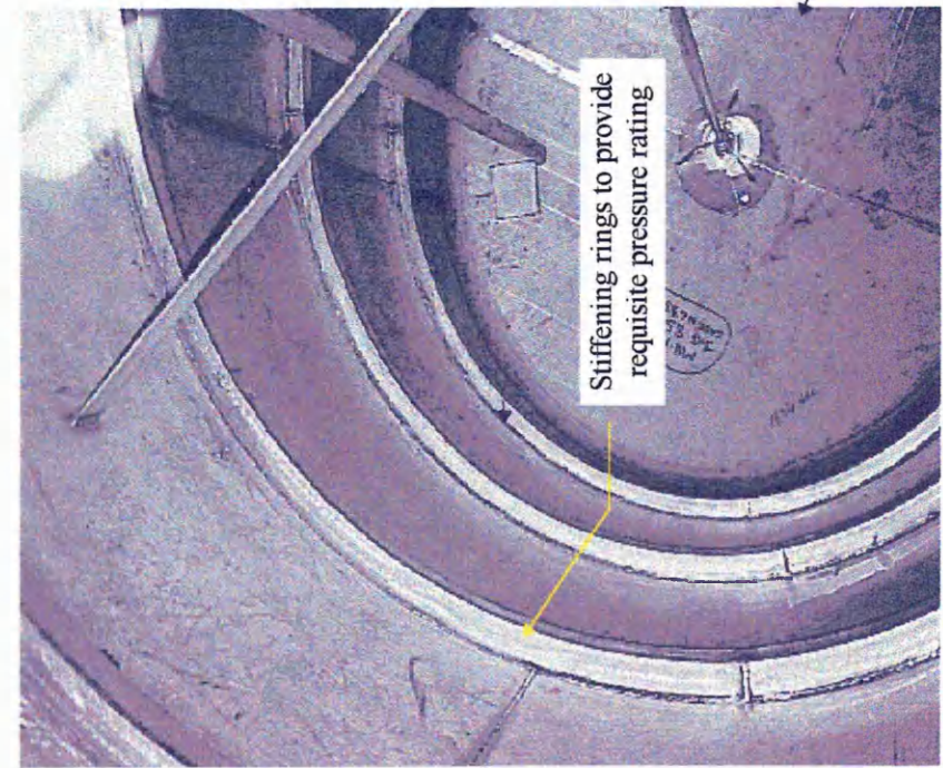
P 13 Internal photograph of DMS storage vessel
